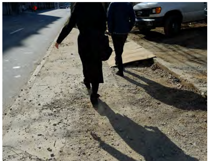
Extensive debris on sidewalk on Spring St
