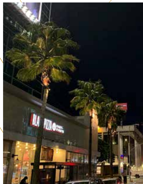
After months of permitting delays, the Sunset Palm up-lights were finally installed in February.
