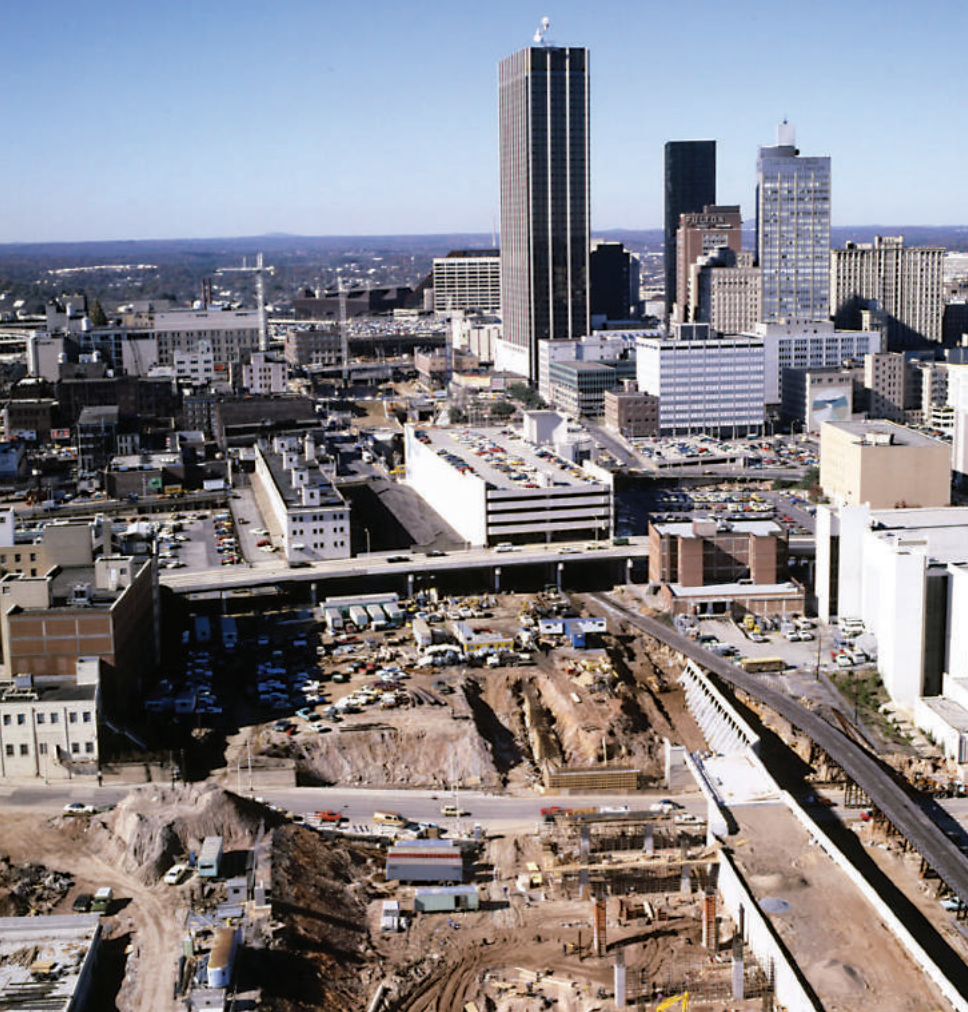
Construction of the MARTA East Line, Downtown Atlanta, 1977. Source: Atlanta Journal-Constitution Photographic Archives. Special Collections and Archives, Georgia State University Library.
