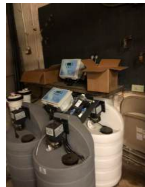
Photo 6 – Chemical Treatment System
