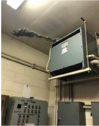
Photo 7 – Transformer and Electric
