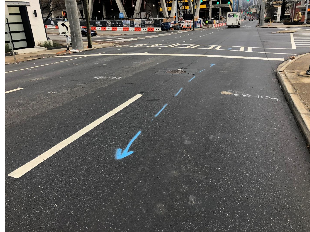
B-10 AREA - LEVEL 2 FATIGUE CRACKING, RAVELLING
