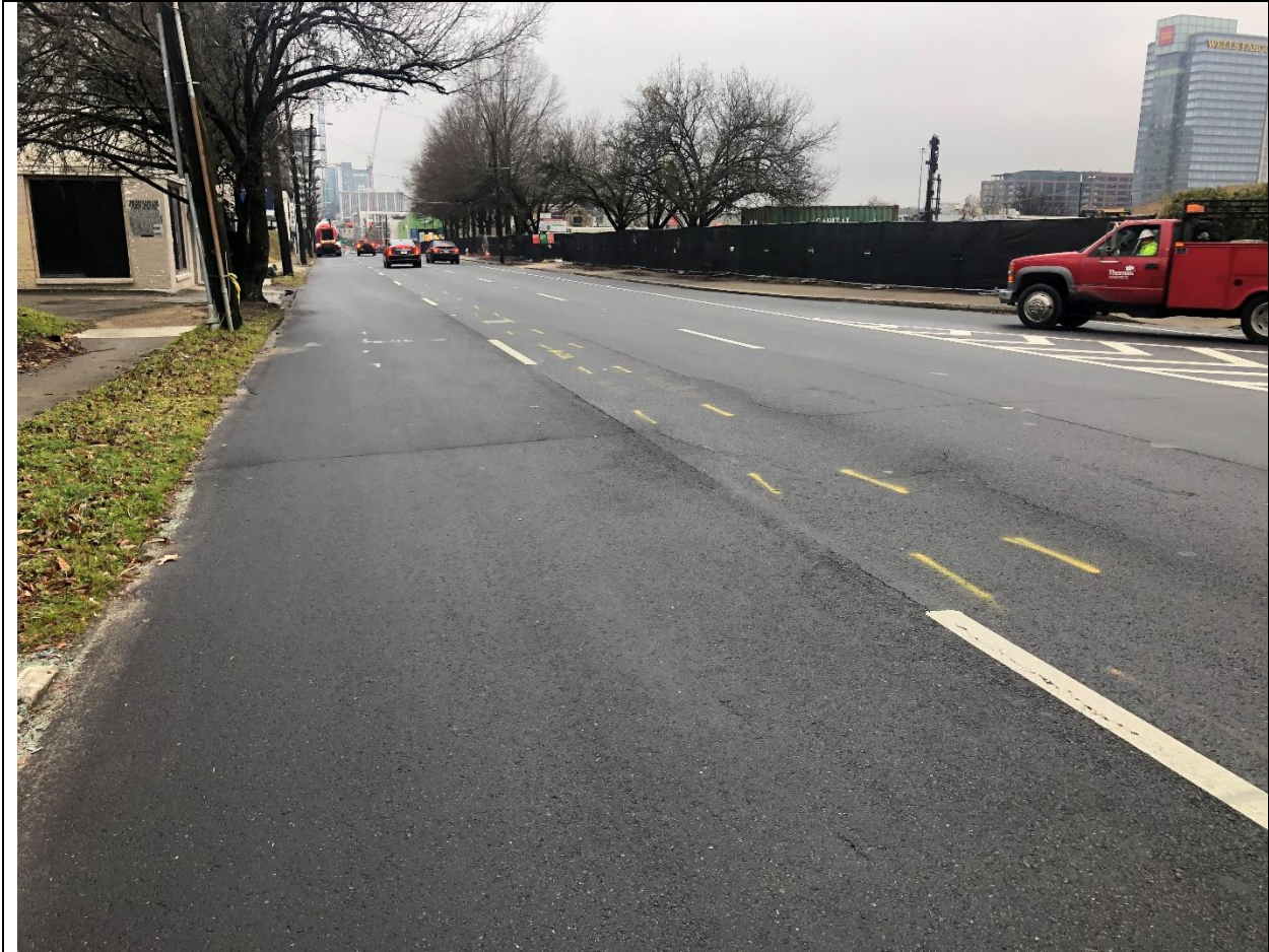
B-4 AREA - LEVEL 1 LONGITUDINAL AND TRANSVERSE REFLECTIVE CRACKING, RAVELLING
