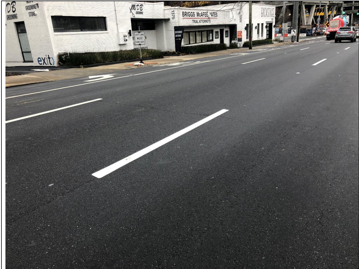
B-8 AREA - LEVEL 1 LONGITUDINAL AND TRANSVERSE REFLECTIVE CRACKING
