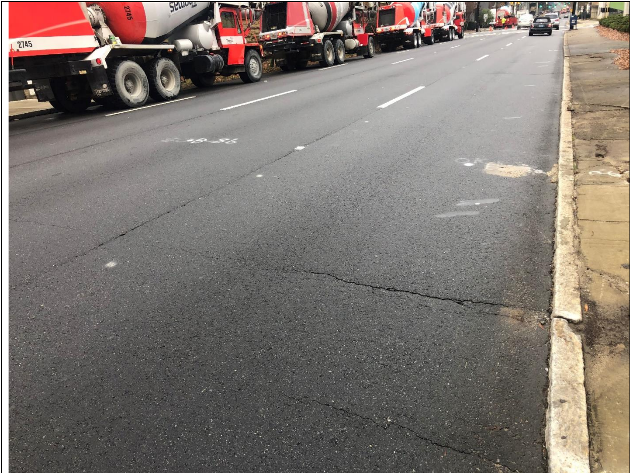
B-8 AREA - LEVEL 2 LONGITUDINAL AND TRANSVERSE REFLECTIVE CRACKING
