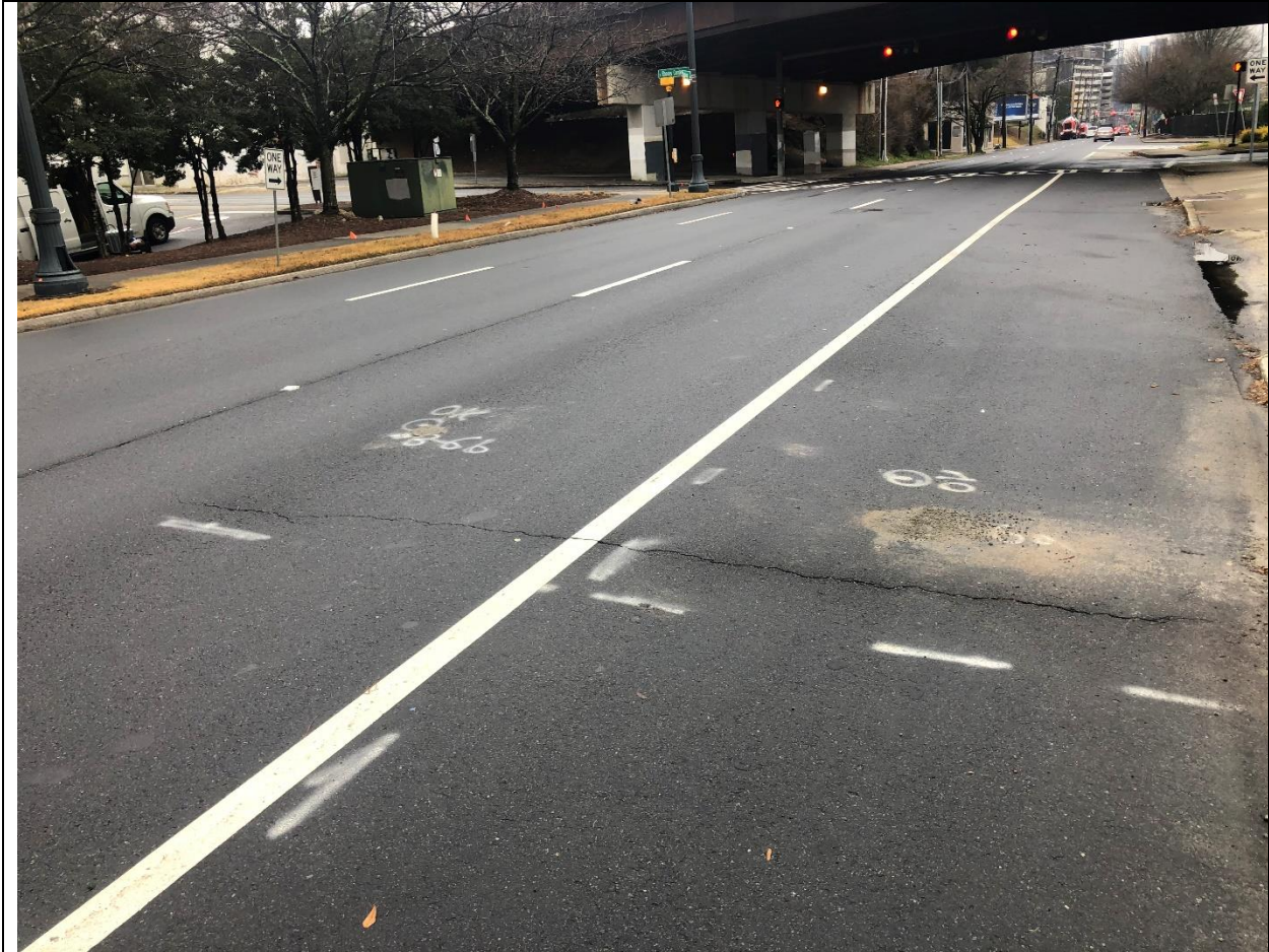
B-6 AREA - LEVEL 1 LONGITUDINAL/ TRANSVERSE REFLECTIVE CRACKING
