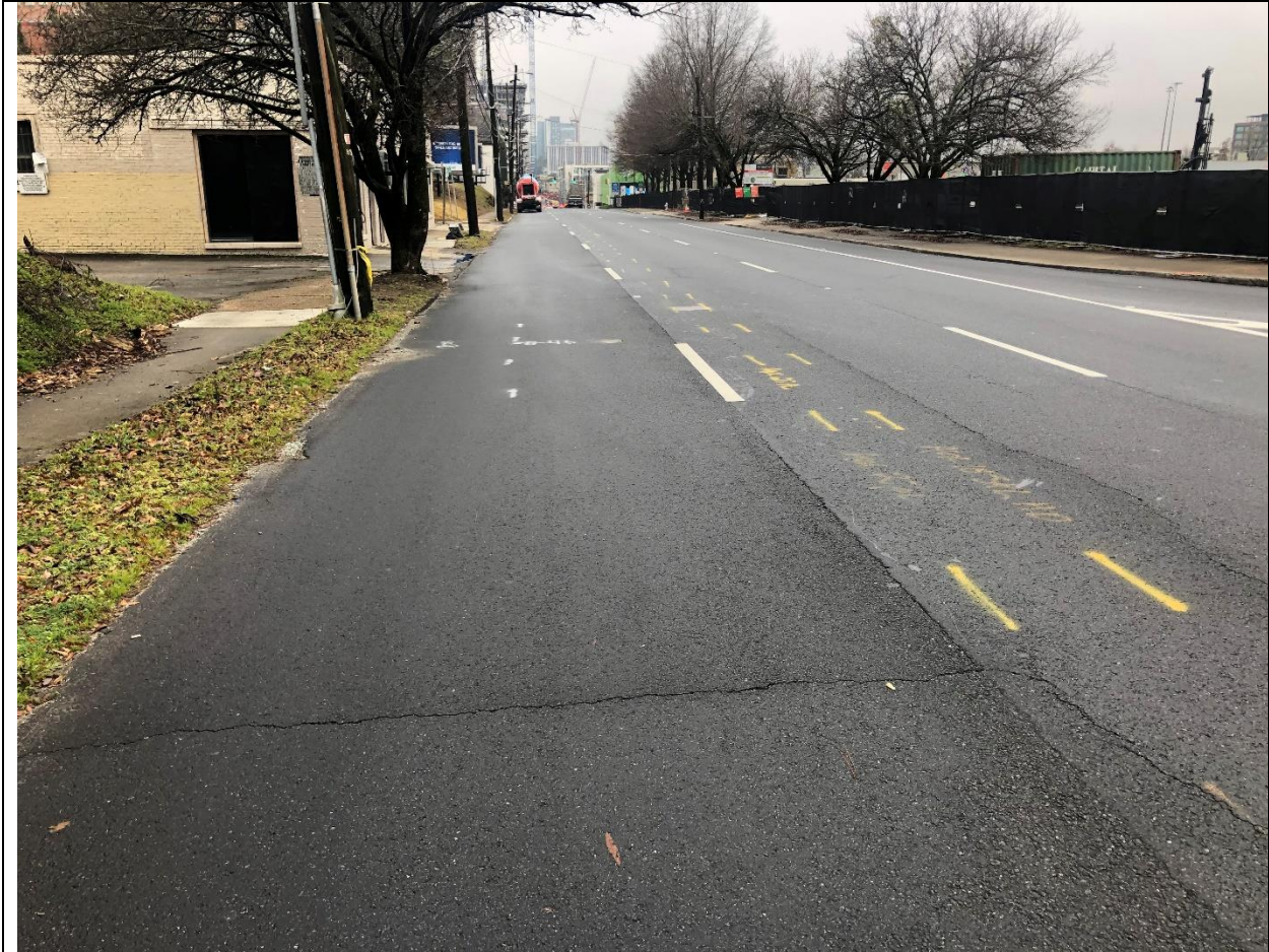
B-4B AREA - LEVEL 1 LONGITUDINAL AND TRANSVERSE REFLECTIVE CRACKING
