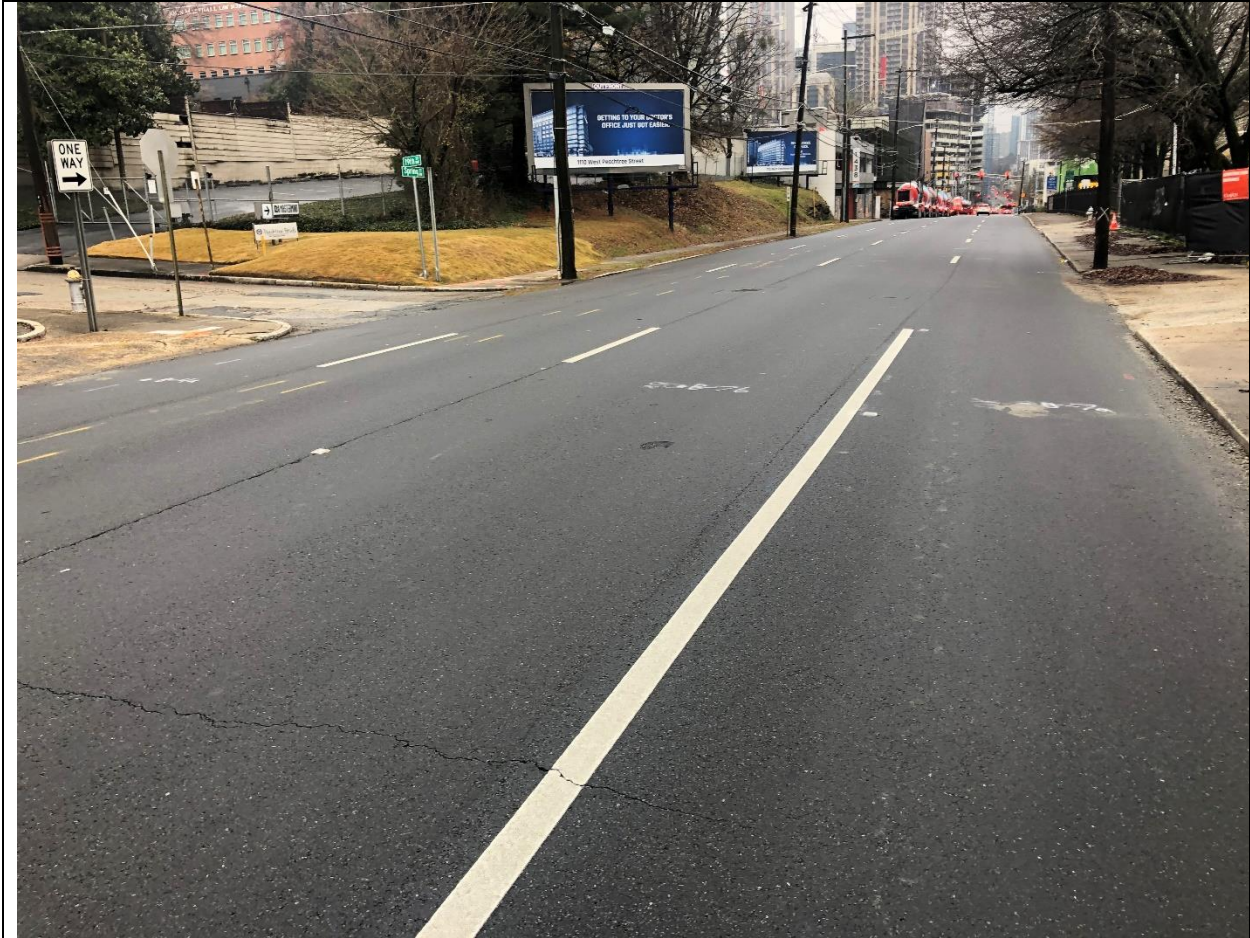
B-7- AREA - LEVEL 1 LONGITUDINAL AND TRANSVERSE REFLECTIVE CRACKING
