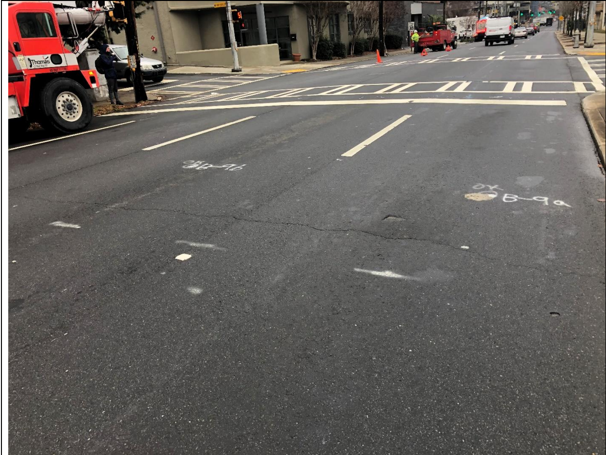
B-9 AREA - LEVEL 1 LONGITUDINAL AND TRANSVERSE REFLECTIVE CRACKING, RAVELLING
