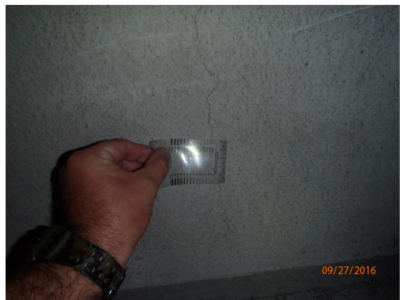
Team C 9-27-16, Cracking in columns up to .006" wide
