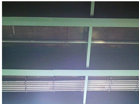
COMMUNICATION AND GAS
