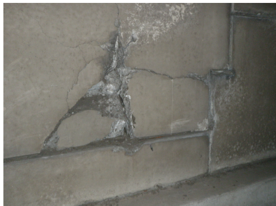
Accident damage on abutment 4 wall.
