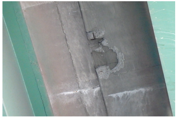
Deck spall span #1bottom
