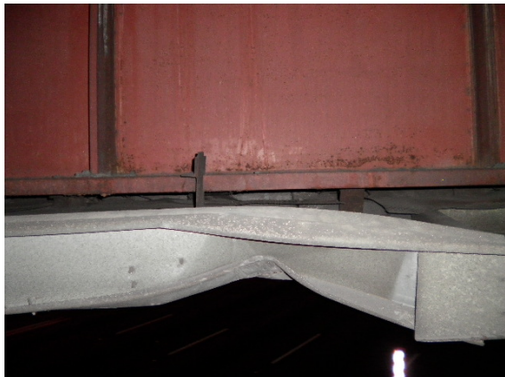
Collision damage span 1 over right lane, broken panels and panel supports (Beam 3-5).
