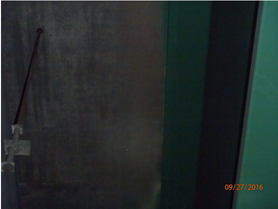
Team C 9-27-16, Cracking in deck underside up to .008" wide with efflorescence
