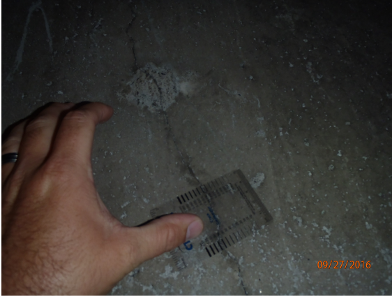
Team C 9-26-16, Vertical cracking in pier wall 2 up to .025" wide
