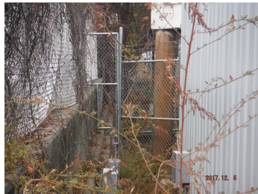
Figure A-4: Proximity of The Old New York 19 Condo Foundation to Wall N
