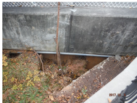
Figure A-6: Soil Erosion Behind Wall N
