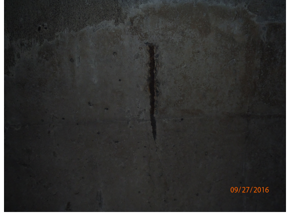
Team C 9-26-16, Pier wall 2 spall with exposed rebar
