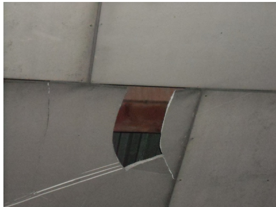
Broken panels span 2, collision damage.
