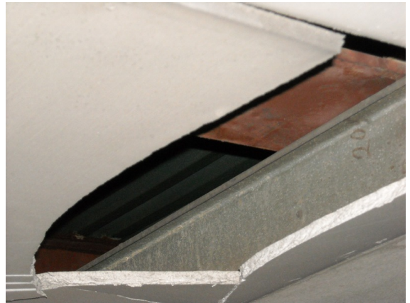
Broken panels span 2, collision damage.
