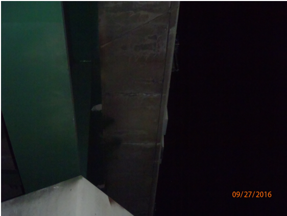
Team C 9-27-16, Cracking in deck overhang up to .005" wide
