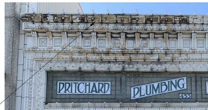
DETAIL AT DETERIORATED TERRA COTTA MASONRY
