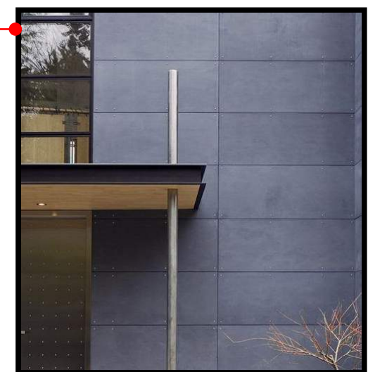
Hardie Panel with exposed fasteners
