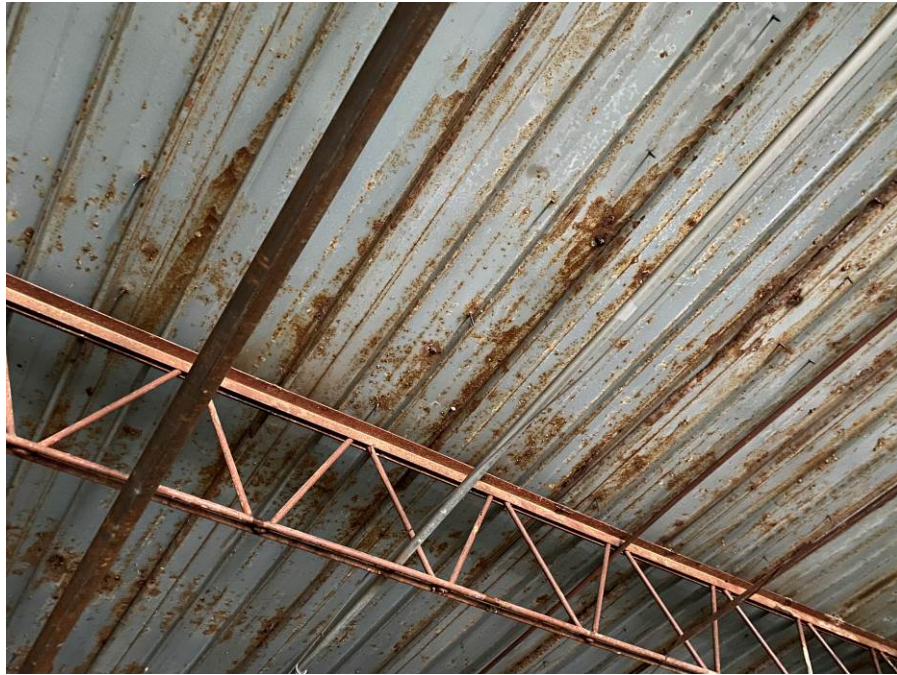
Photo 63 Oxidation Damages on Metal Decking
