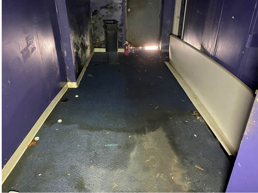
Photo 77 Saturated Floor Framing on 86 North Main
