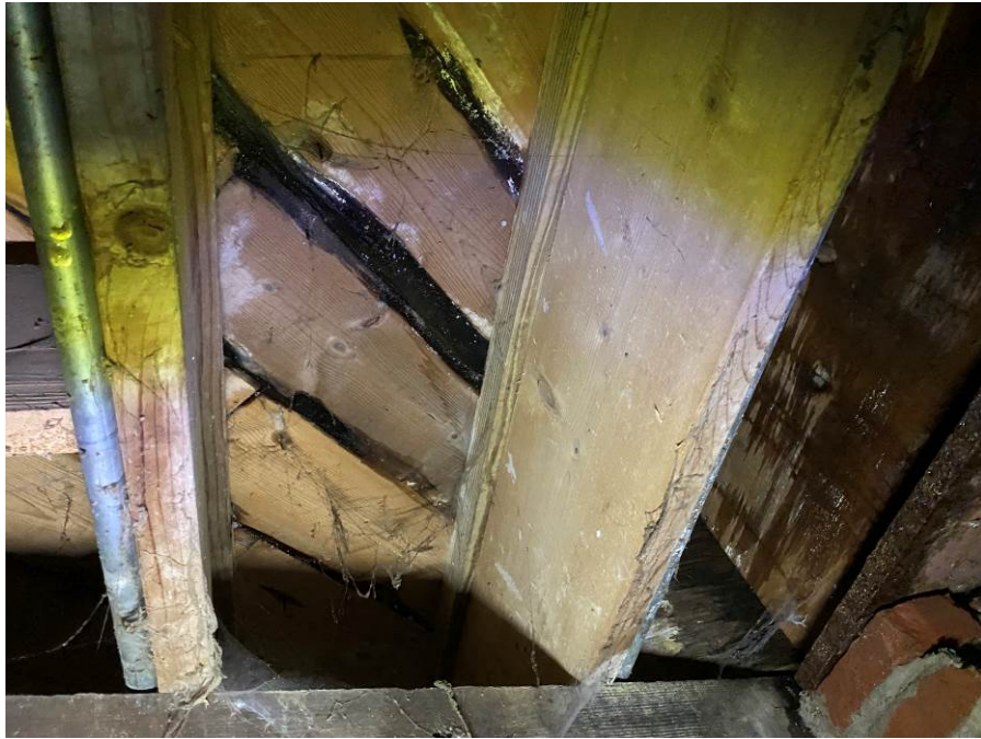
Photo 83 Moisture Damage to Decking at 86 North Main Rear
