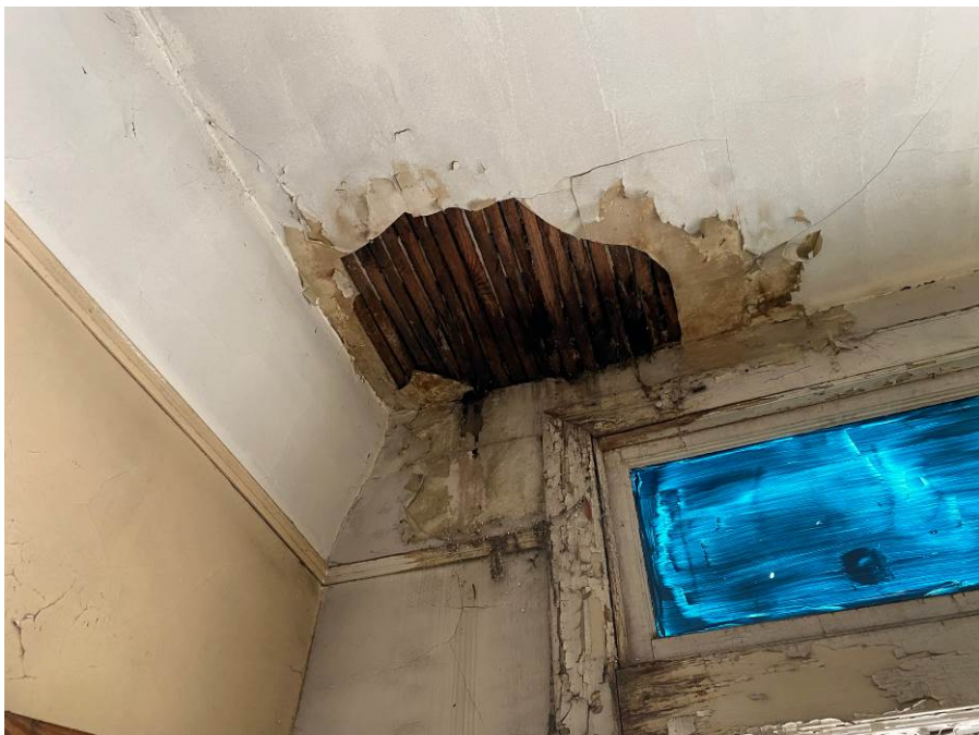
Photo 104 Water Damages in Ceiling of 84 North Main
