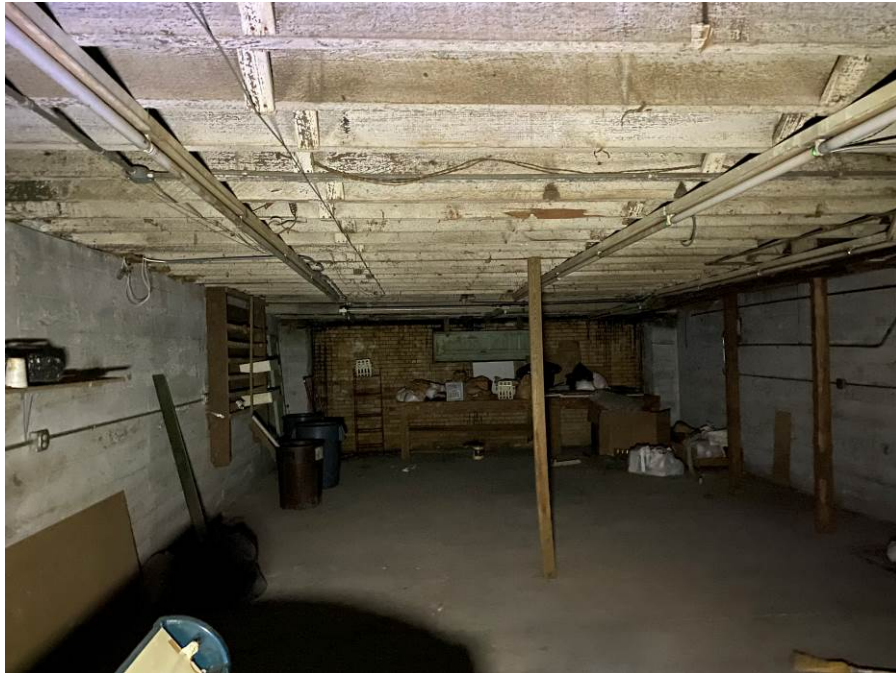
Photo 27 Basement Condition of 84 North Main
