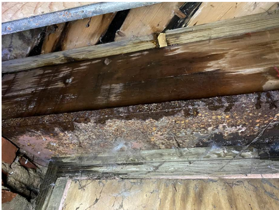
Photo 82 Active Moisture Leak at Framing at 86 North Main
