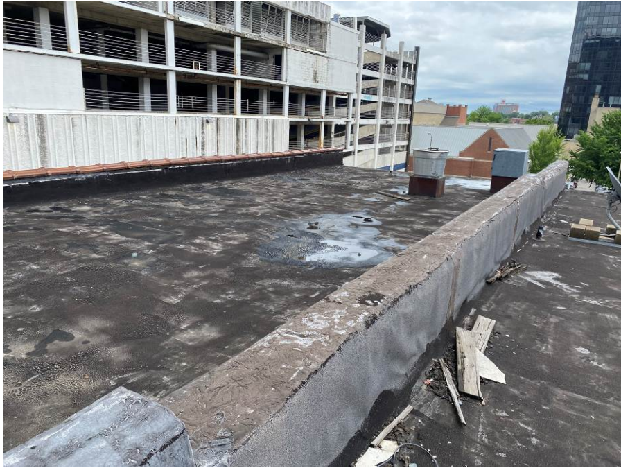
Photo 59 Aged Condition of Roof Coverings
