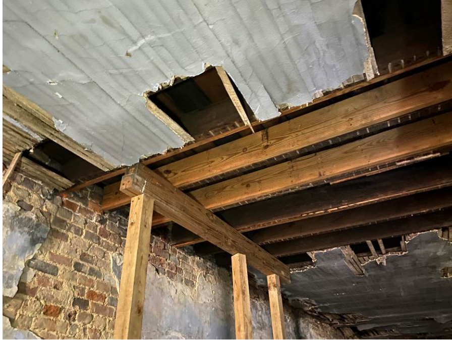
Photo 97 Condition of Existing Shoring at Roof of 86 North Main (Repairs Required)
