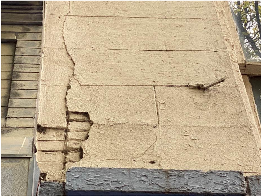
Photo 115 Cracking Parge Coating
