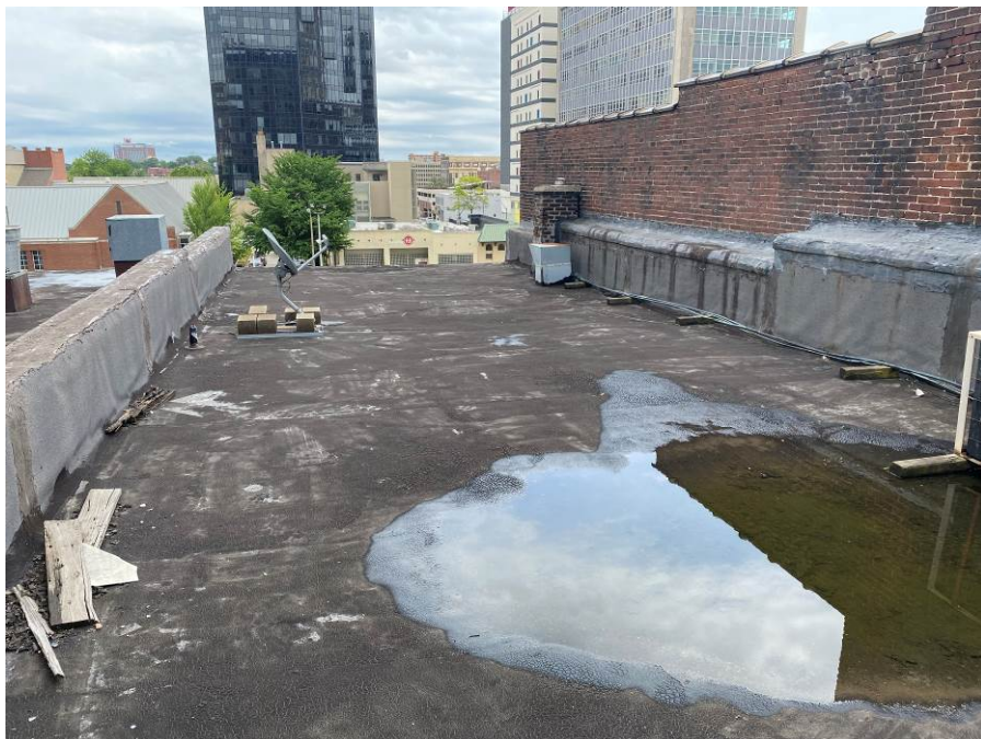
Photo 92 Roof Ponding at 86 North Main
