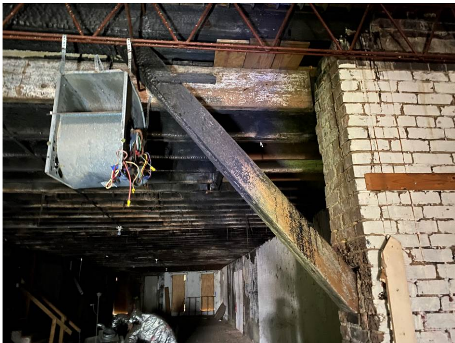
Photo 76 Charred Kicker to be Replaced at 88 North Main
