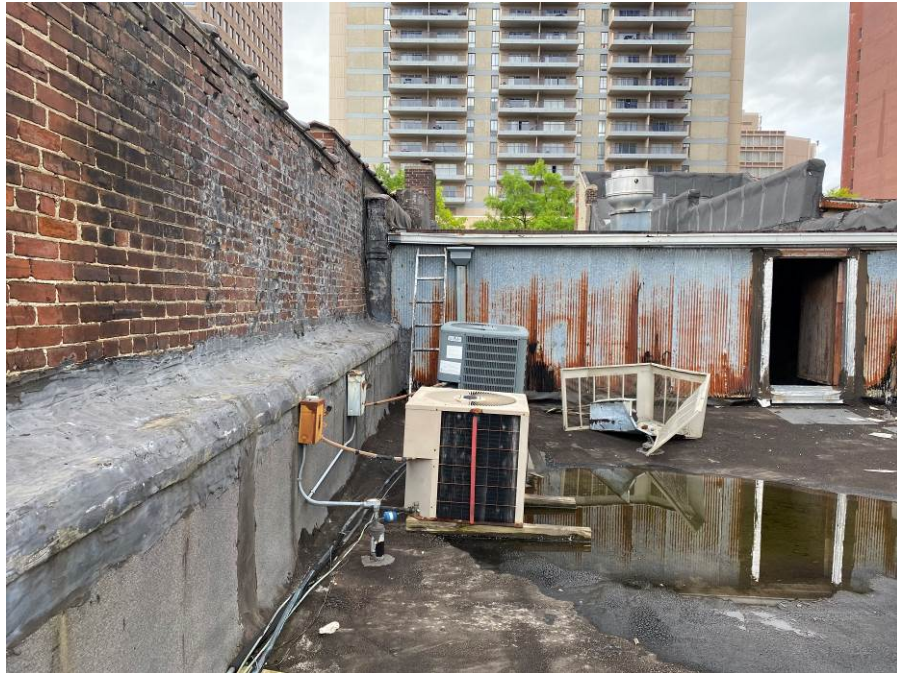
Photo 95 Aged Roof Flashing at Roof Coverings
