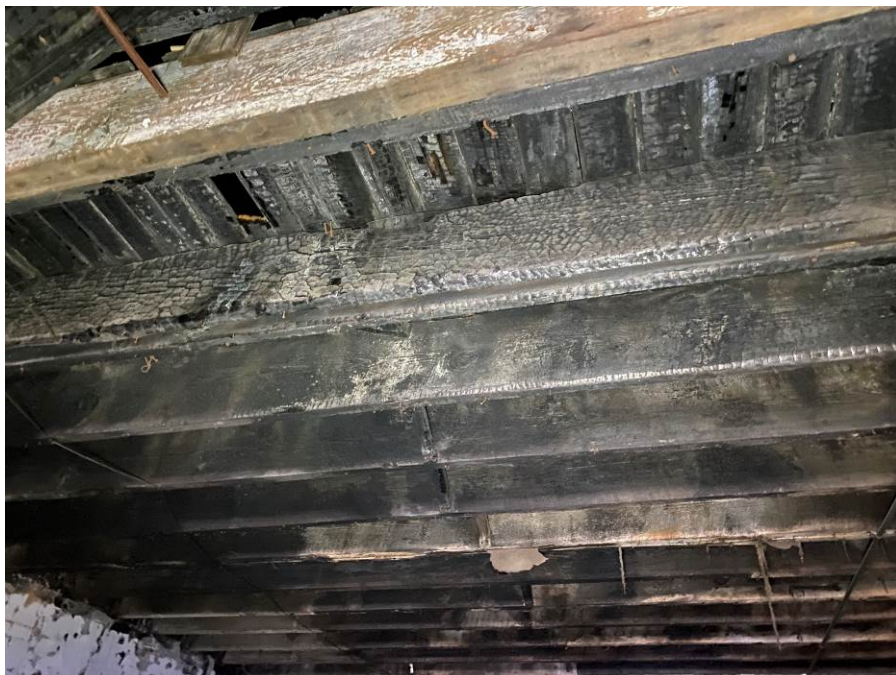
Photo 74 Charred Joists at 88 North Main to be Repaired
