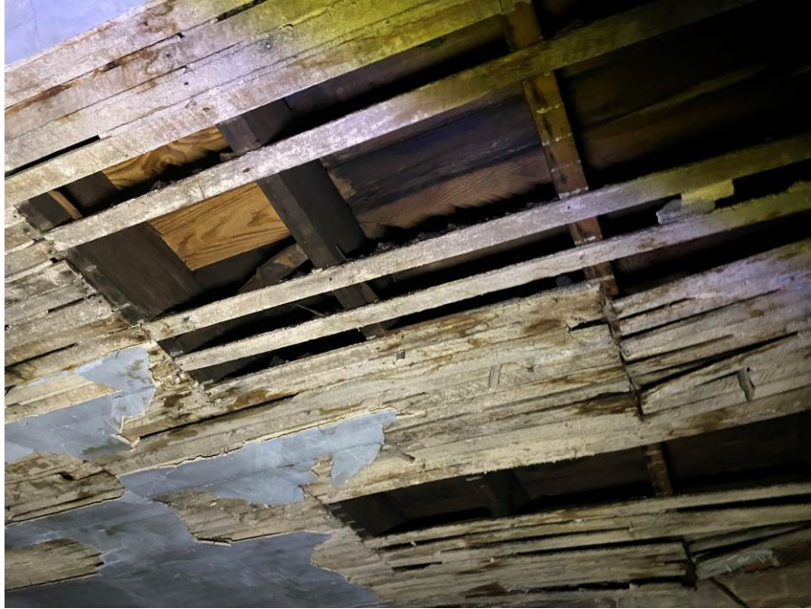
Photo 91 Moisture Damages at 86 North Main Roof to be Repaired
