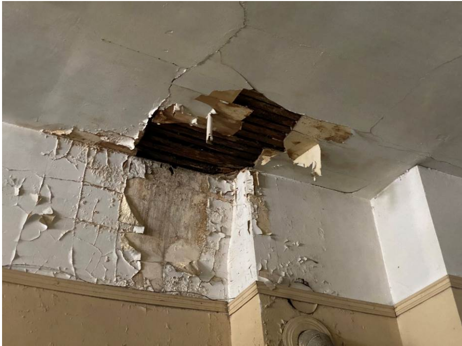
Photo 107 Water Damages to Ceiling and Lath of 84 North Main
