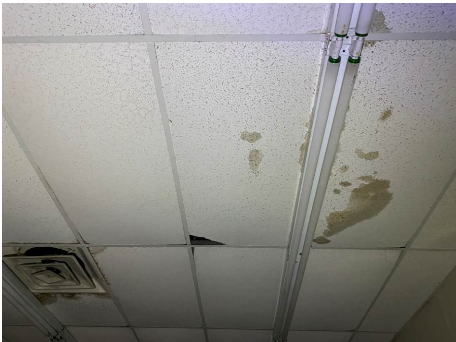
Photo 102 Acoustical Ceiling Tile Water Stains at 84 North Main
