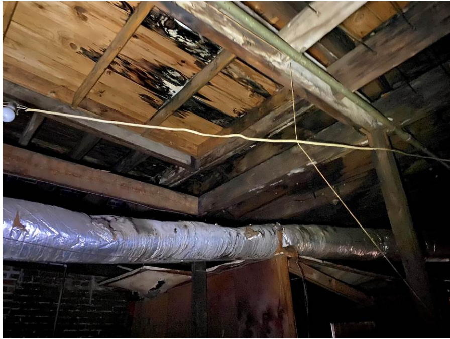
Photo 85 Roof Decking Moisture Damages on 86 North Main
