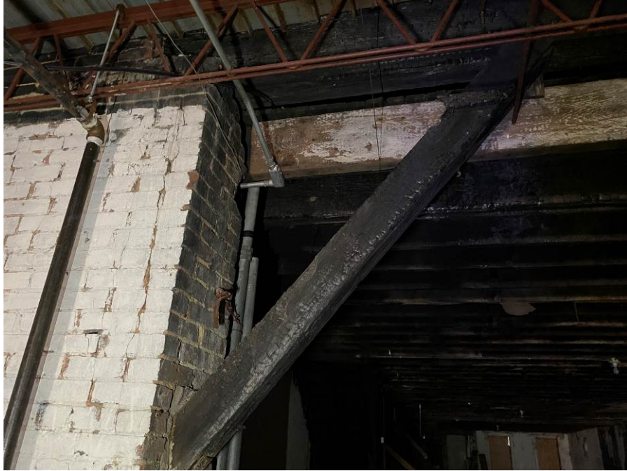
Photo 75 Charred Kicker to be Replaced on 88 North Main
