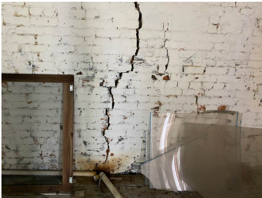
Photo 42 Magnitude of Masonry Crack on 88 North Main
