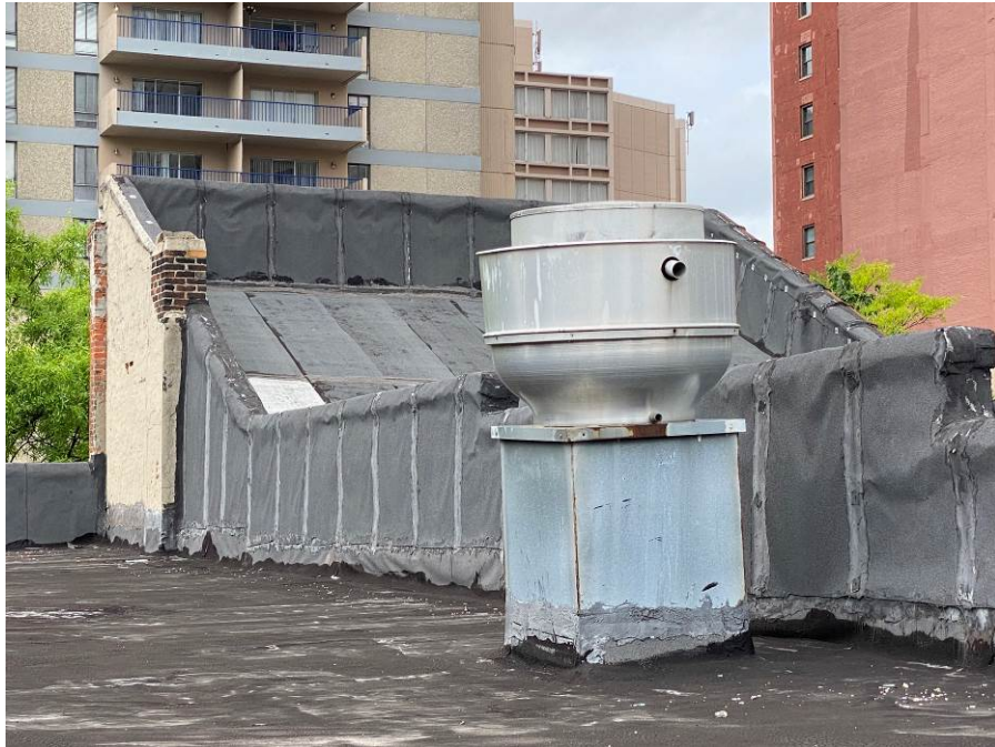
Photo 65 Four Story Roof Area with Aged Roof Coverings on 88 North Main
