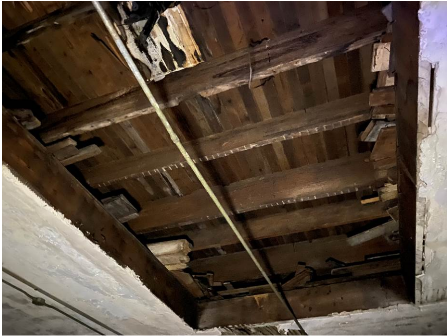
Photo 117 Decking Water Stain Damages at Roof of 80 North Main
