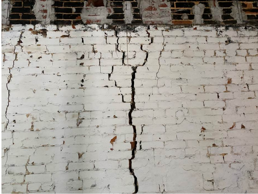
Photo 43 Crack on North Exterior Wall of 88 North Main
