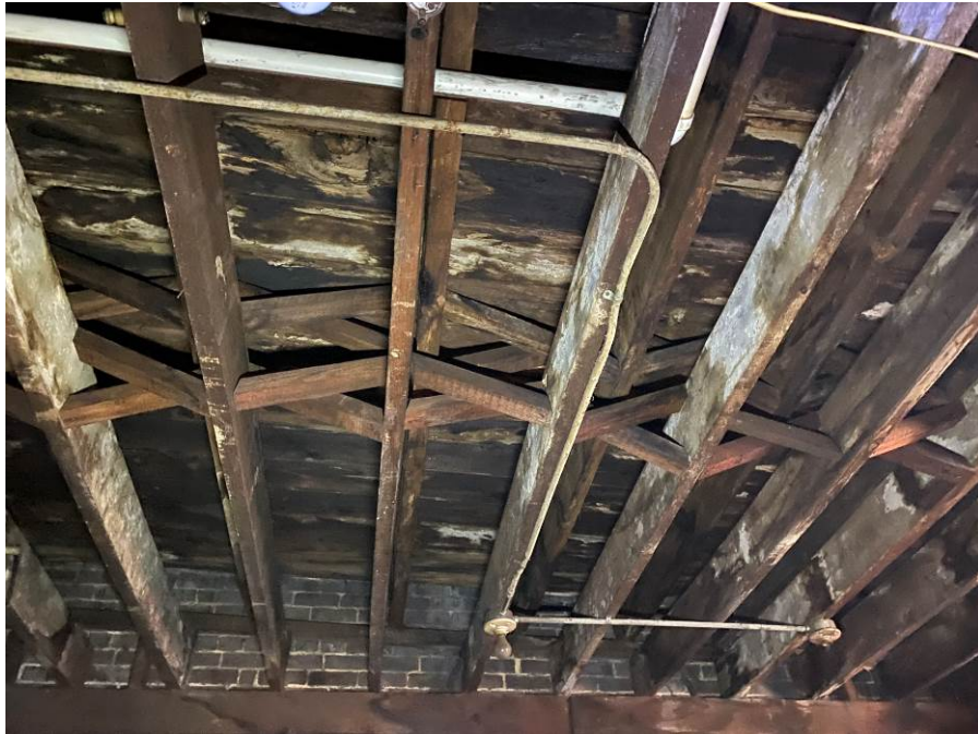
Photo 87 Moisture Exposure to Decking and Framing at Roof at 86 North Main
