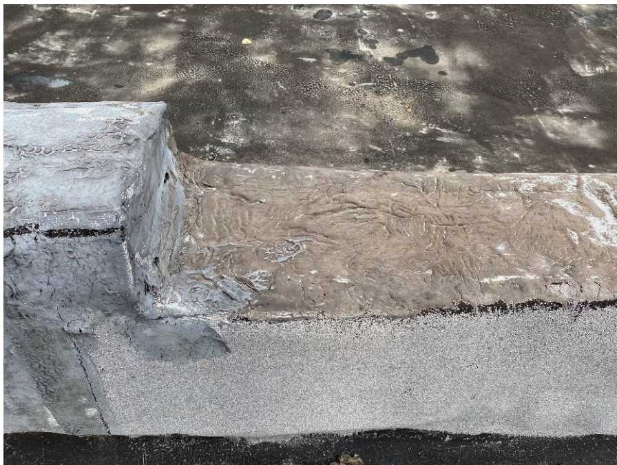
Photo 60 Poor Condition of Wall Flashing Between 88 North Main and 86 North Main
