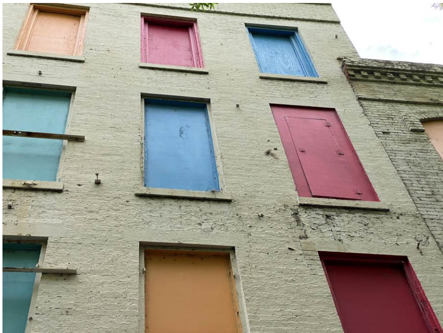
Photo 50 Condition of Exterior Masonry on 88 North Main
