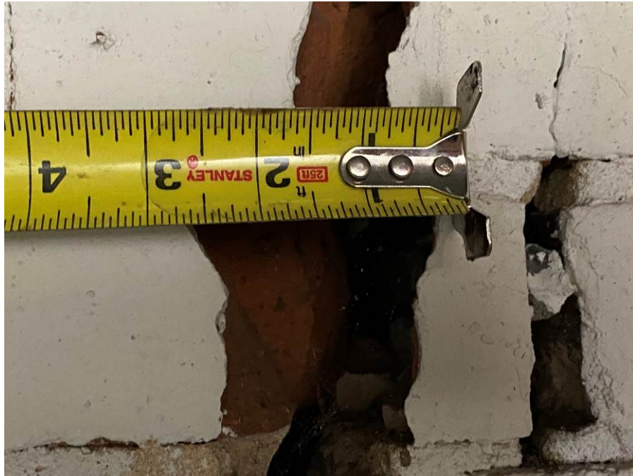
Photo 45 Magnitude of Crack on 88 North Main
