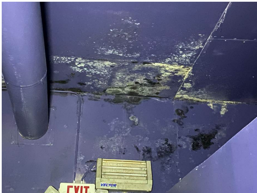
Photo 78 Microbial Growth on Interior Finishes on 86 North Main
