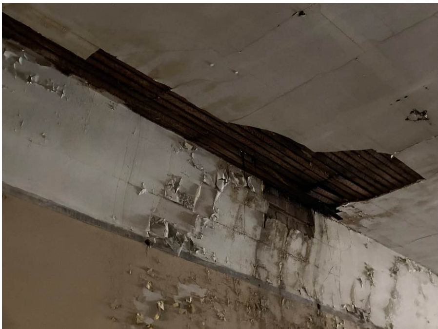
Photo 108 Water Damages to Ceiling on 84 North Main
