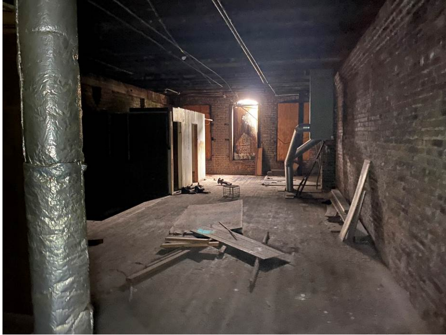
Photo 19 86 North Main General Conditions
