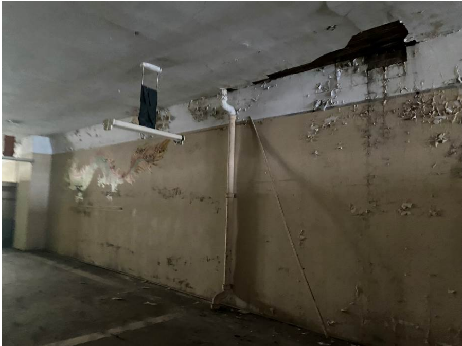
Photo 103 Water Exposure Damage to Covered Ceiling of Second Floor at 84 North Main
