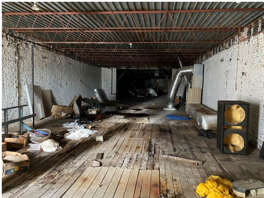
Photo 46 Second Floor Metal Deck and Steel Bar Joists Framing on 88 North Main
