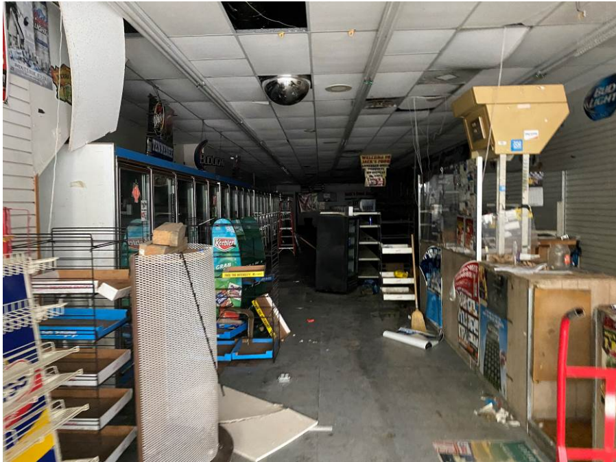
Photo 101 Interior Water Stains to Acoustical Ceiling Tiles at 84 North Main
