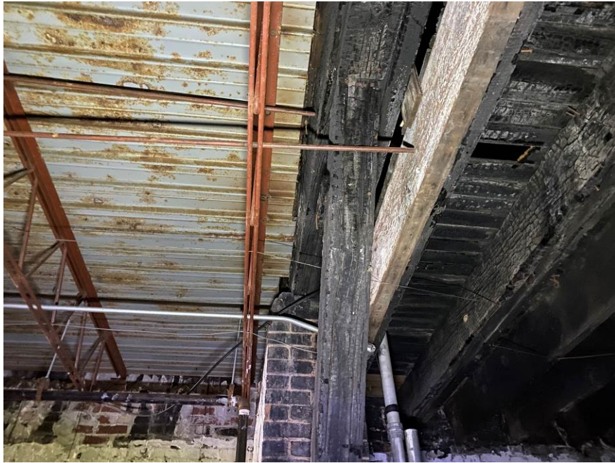
Photo 73 Charred Framing at 88 North Main to be Repaired
