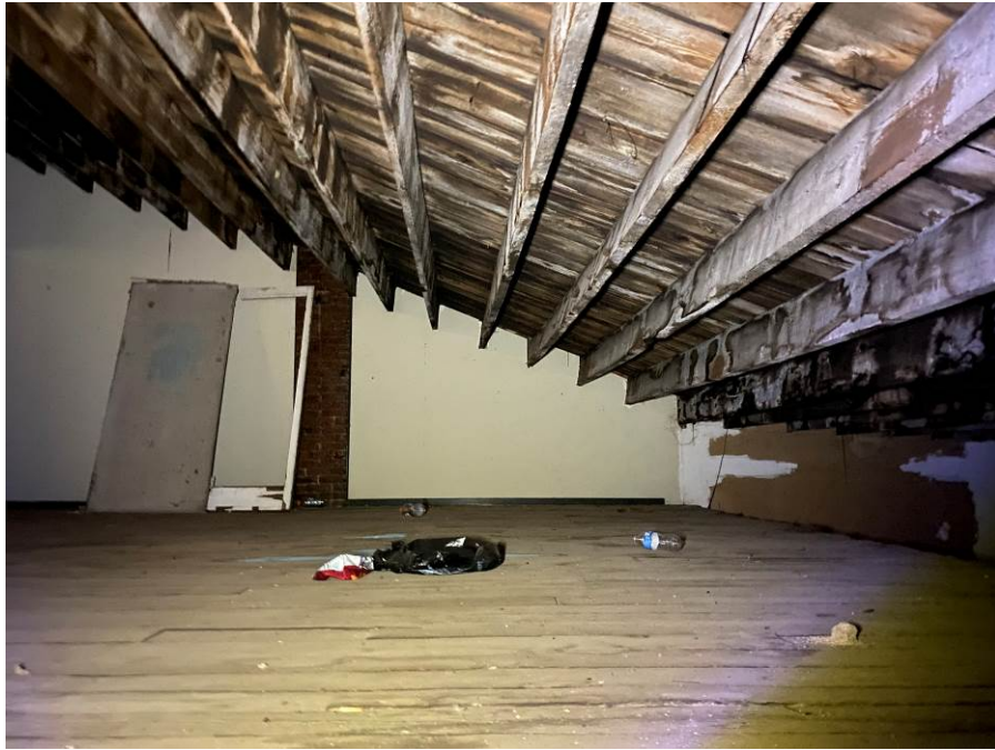
Photo 69 General Condition of the Roof Framing at the Fourth Story Area on 88 N Main
