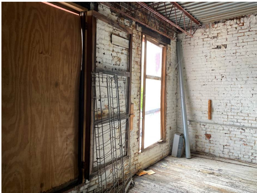
Photo 56 Open Exterior Windows and Openings at 88 North Main
