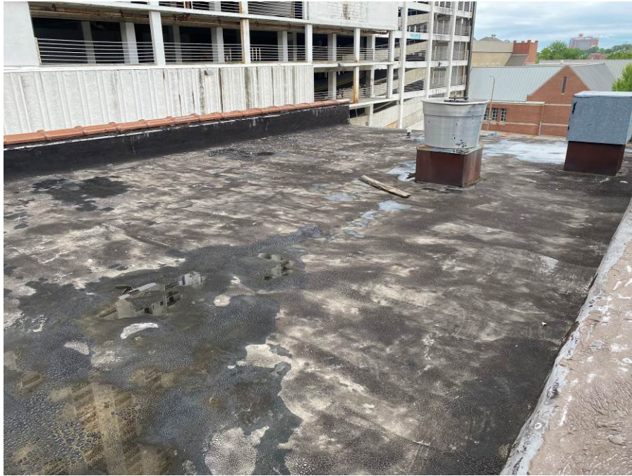
Photo 61 Ponding over 88 North Main
