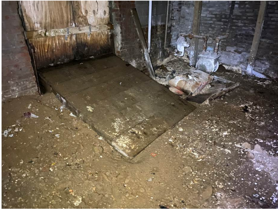
Photo 79 Water Entry into 86 North Main Basement
