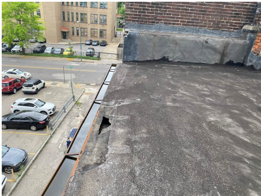
Photo 94 Gutters Full and Hole in Roof Coverings at 86 North Main
