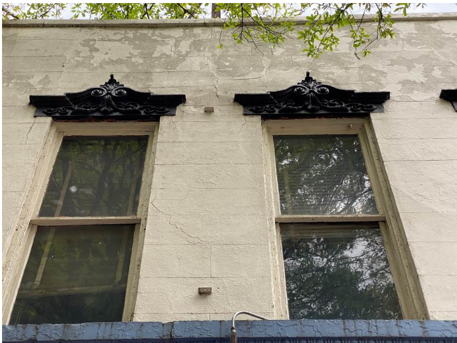
Photo 114 Parge Coat Cracking on Facade
