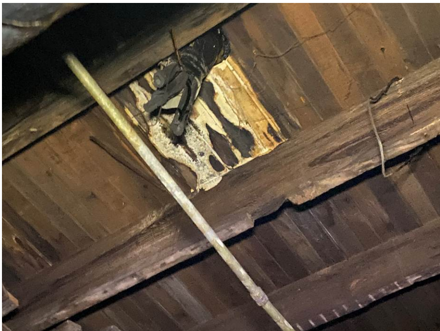
Photo 118 Water Stain Damages at 80 North Main
