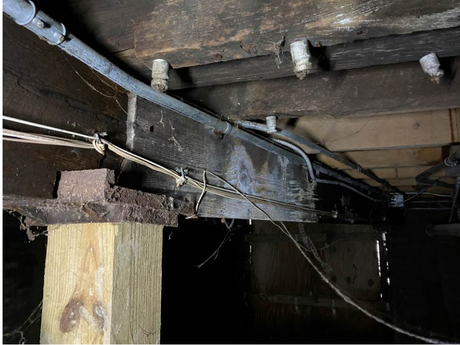
Photo 81 Moisture Stains on Framing in Basement of 86 North Main
