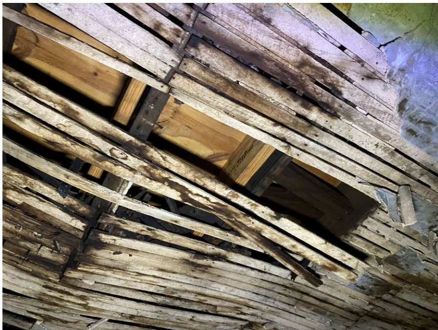
Photo 90 Lath Ceiling Moisture Damage at 86 North Main
