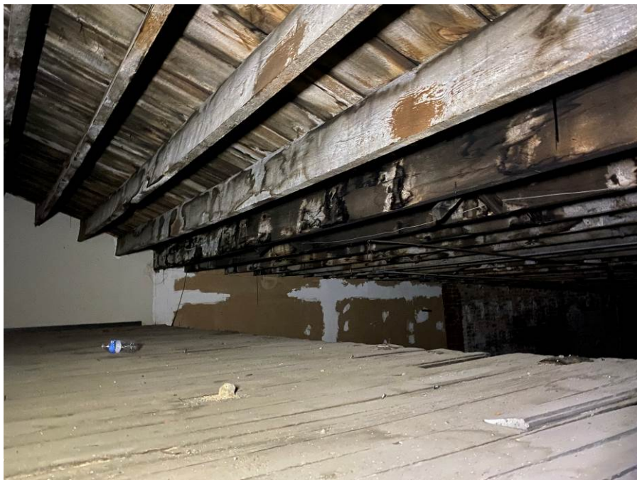
Photo 68 Condition of Roof Joists at 88 North Main Four Story Area
