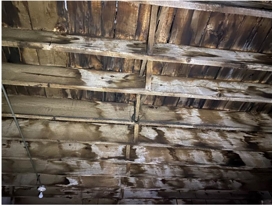
Photo 67 Roof Joists Condition at 88 North Main (Water Staining Damages)
