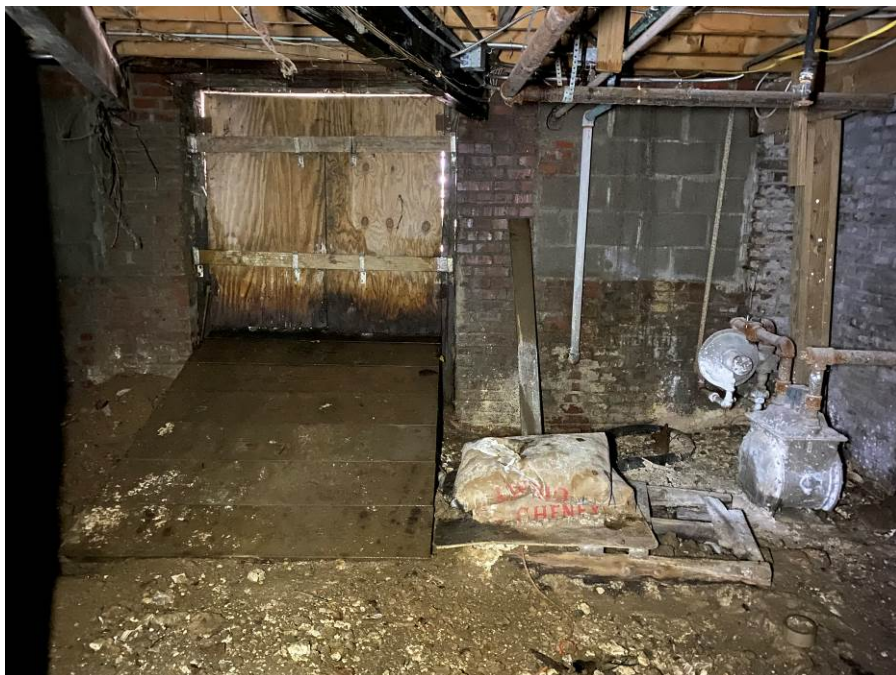
Photo 80 Water Entry into the Basement of 86 North Main
