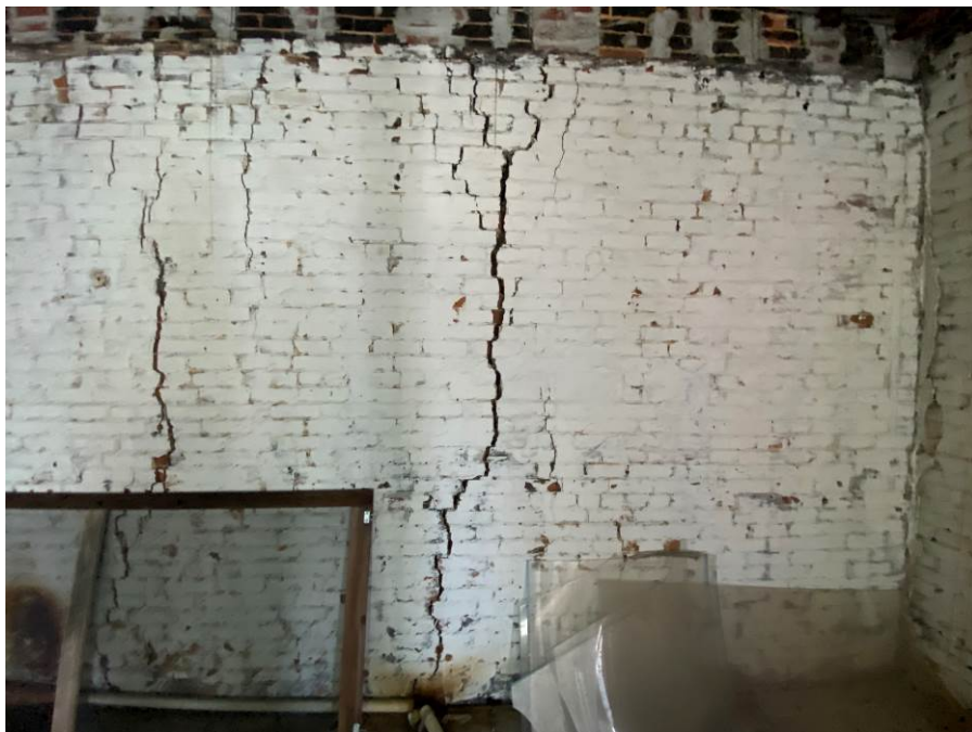
Photo 44 Exterior Wall Cracks on 88 North Main
