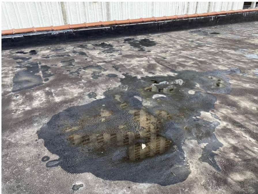
Photo 62 Ponding on Roof Coverings
