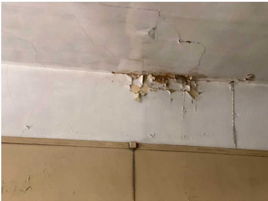
Photo 106 Water Exposure Damages to 84 North Main
