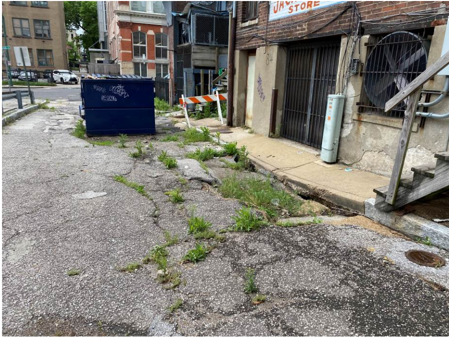
Photo 109 Collapsing Sidewalk and Pavement of November 6 th Alley
