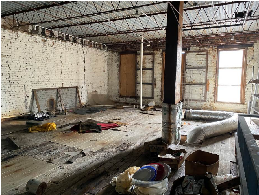
Photo 41 Masonry Crack on 88 North Main
