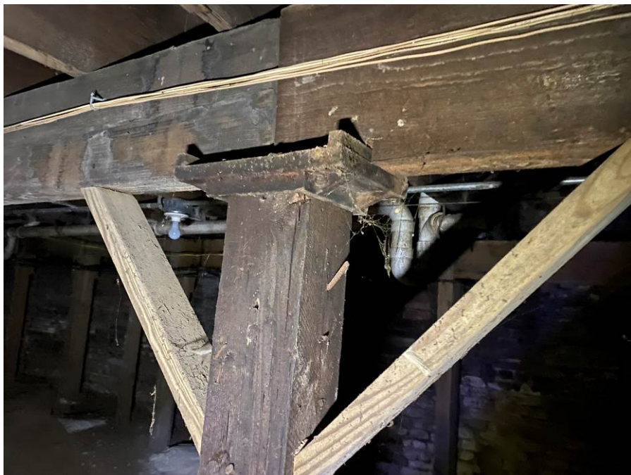
Photo 16 General Connections at Basement in 86 North Main Basement
