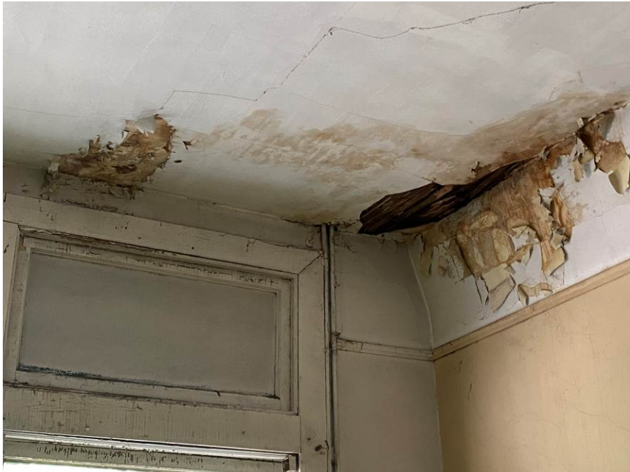
Photo 105 Water Damages in Ceiling at 84 North Main
