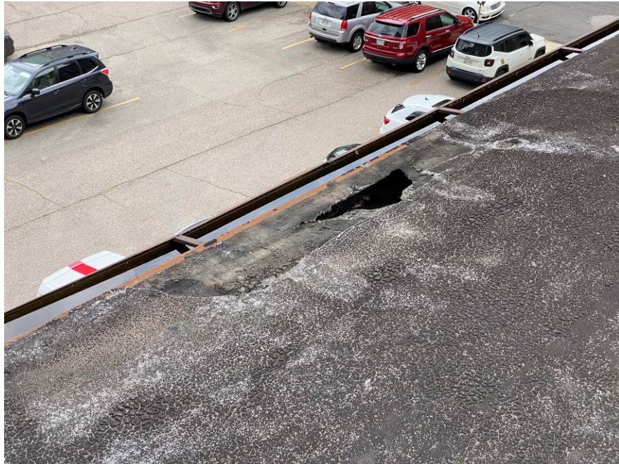
Photo 93 Hole in Roof Coverings on 86 North Main Causing Damages Below
