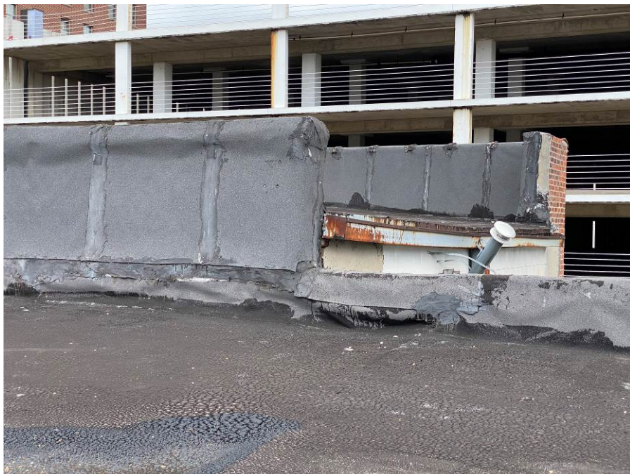
Photo 66 Parapet Wall with Aged Wall Flashing with Gaps and Openings
