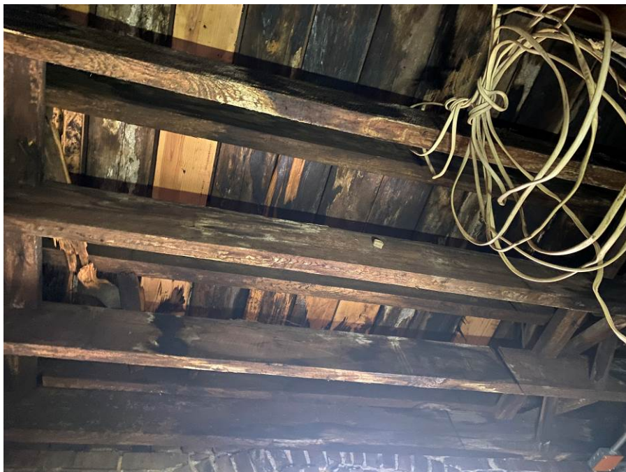
Photo 88 Moisture Damages to Decking at 86 North Main
