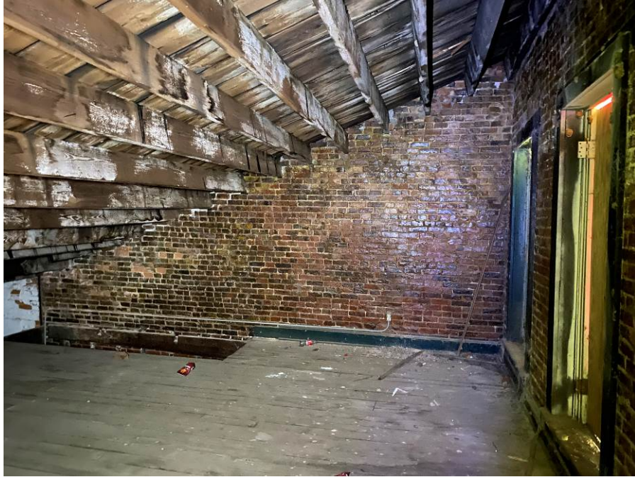
Photo 71 Water Stains on Roof Framing Members on 88 North Main
