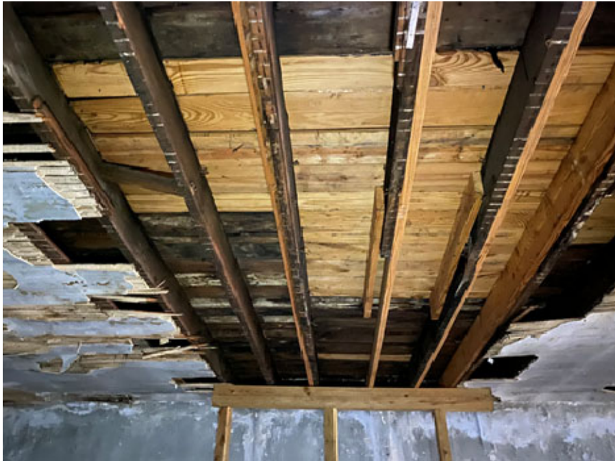
Photo 99 Shoring Condition at 86 North Main Roof (Repairs Required)
