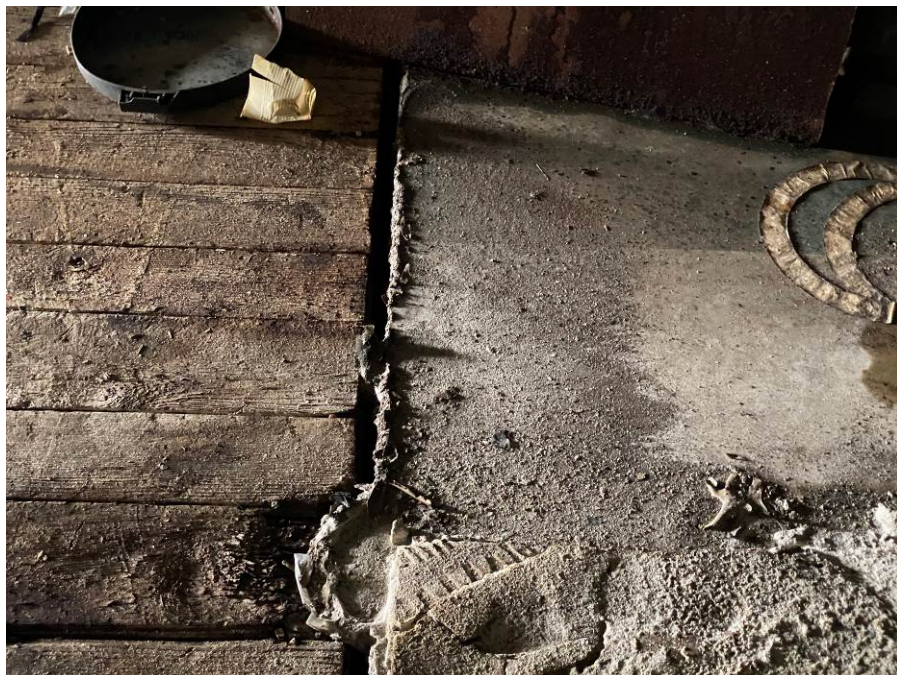
Photo 64 Joint at Concrete and Floor Decking at 88 North Main
