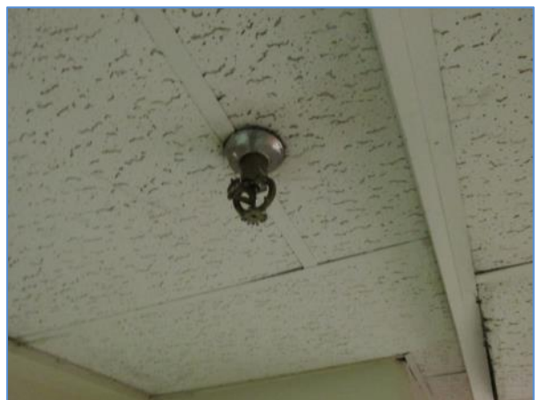
Sprinkler head in the lower lobby
