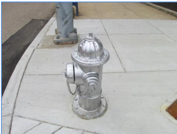
Hydrant in the sidewalk surrounding the site
