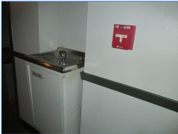
Non-compliant water fountain in a common hallway on an upper floor
