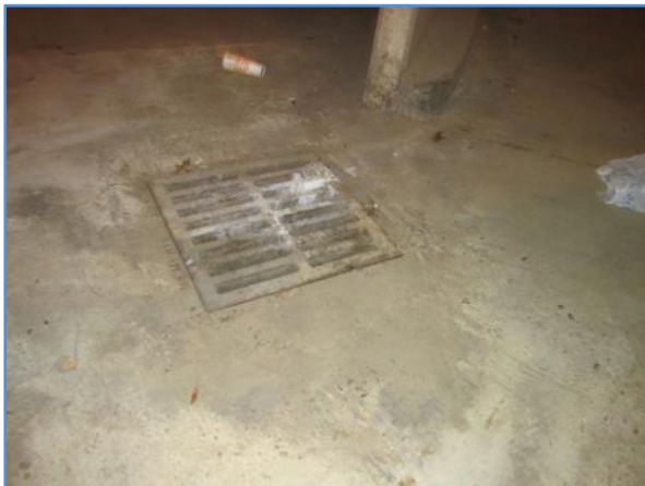
Area drain in the parking garage
