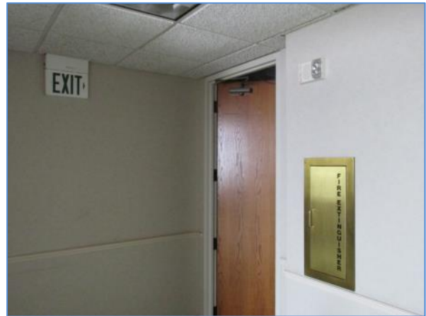
Exit signage, strobe and fire hose in a wall mounted cabinet on the 34 th floor
