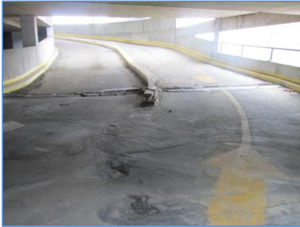
Deteriorated pavement conditions and concrete curbing (center) at the upper garage level ramp
