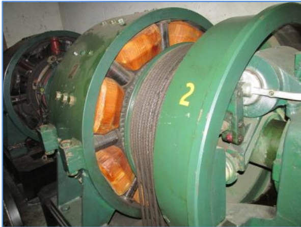
Typical view of the elevator equipment
