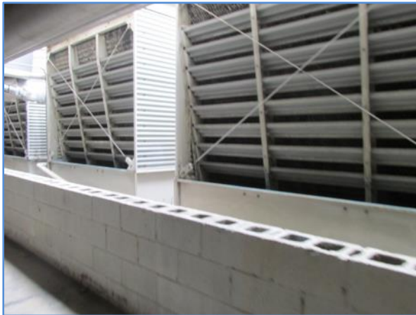
The cooling towers as viewed from the 7 th floor parking deck
