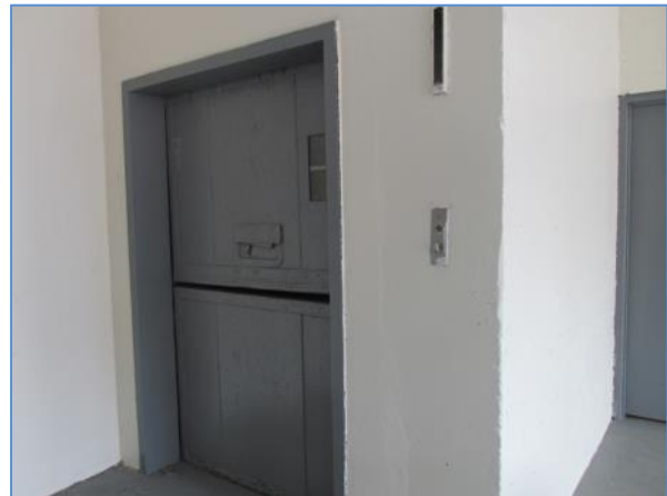
The freight elevator at the loading dock that reportedly accesses the 4 th floor kitchen
