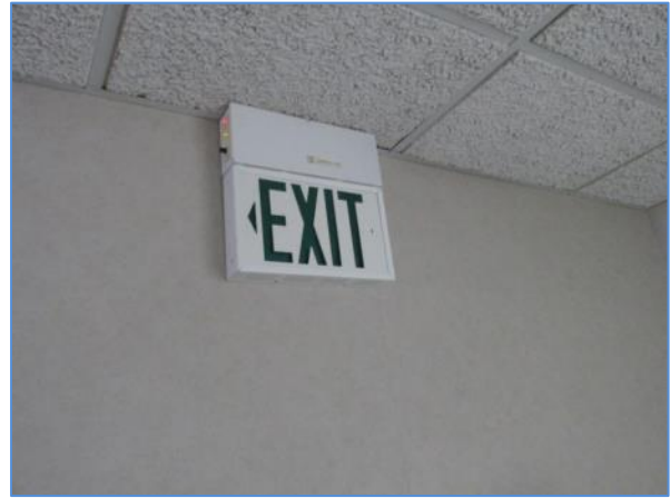
Exit signage on an upper floor
