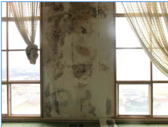
Suspected water damage due to window leaks on the 34 th floor
