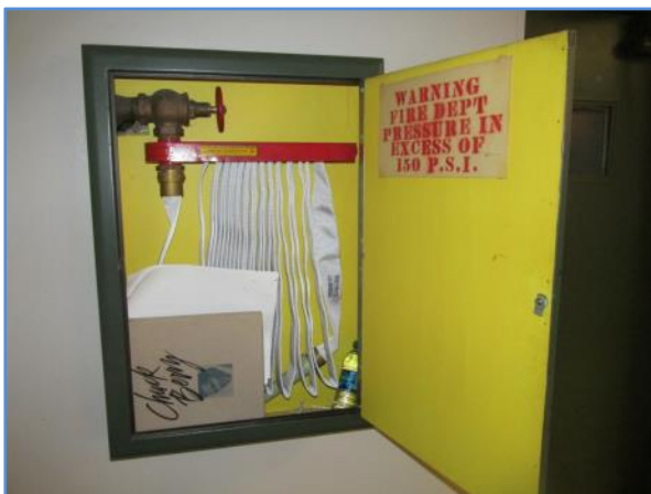
Fire hose in a cabinet at the main lobby on the ground floor
