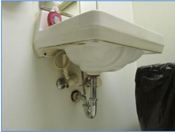
Typical piping beneath a restroom sink
