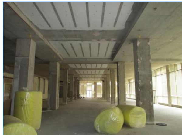
Vacant area on the first floor showing reinforced concrete floors and columns
