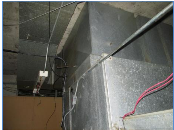
Typical view of an air handler on the floors
