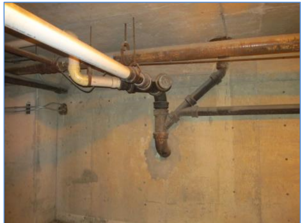
Waste lines in the basement parking garage; note PVC replacement piping
