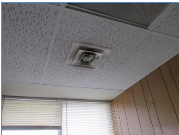
Air diffuser in a vacant office space
