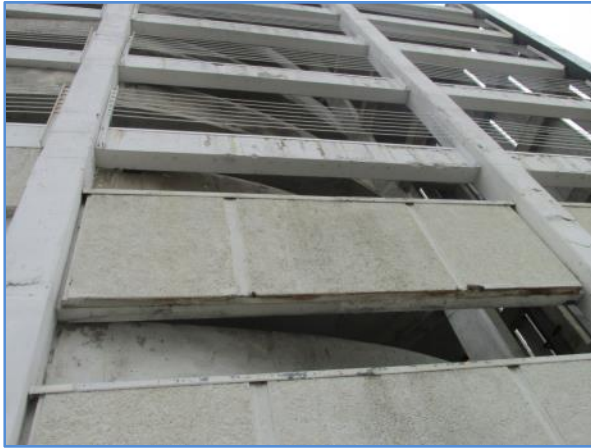
Façade conditions at the south side of the building at the parking garage
