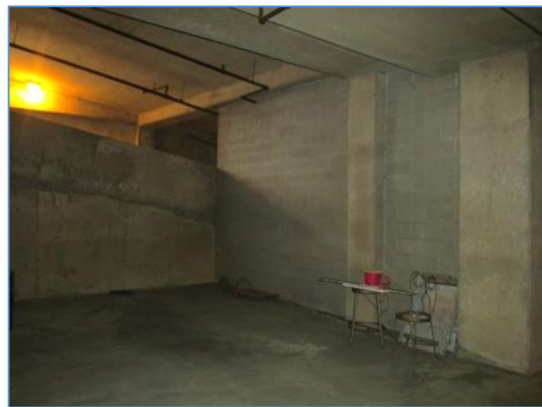
CMU and poured concrete walls in the lower level of the parking garage
