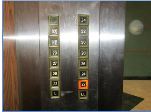
Non-compliant elevator cab panel
