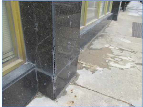
Damage to marble cladding on the lower north facade
