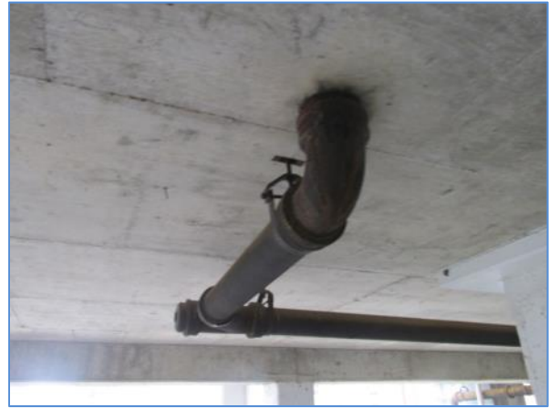
Cast iron drain line at the 7 th floor of the parking garage
