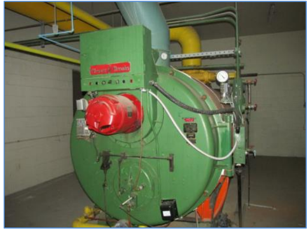
One of the Cleaver Brooks boilers (disconnected) in the 7 th floor mechanical room
