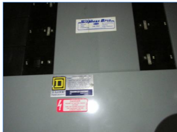
1,200-amp panelboard in the basement electrical room
