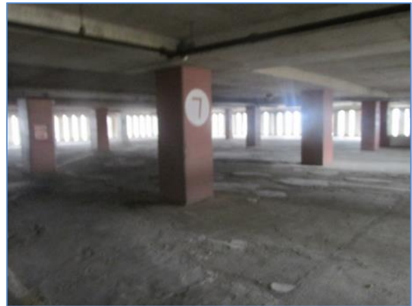
Deteriorated pavement conditions at level 7 of the parking garage
