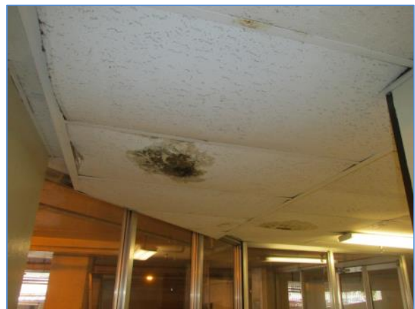
Stained ceiling tile in the lower lobby common corridor
