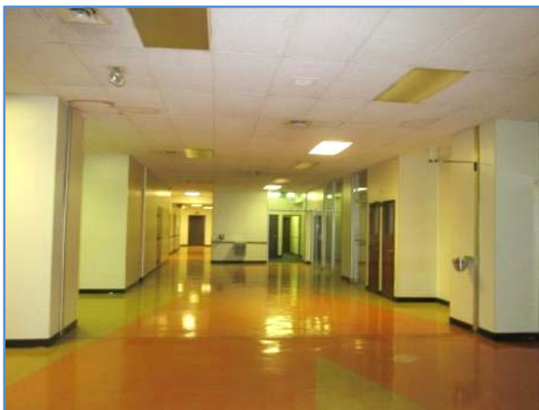
Stained ceiling tiles in the 4 th floor common corridor
