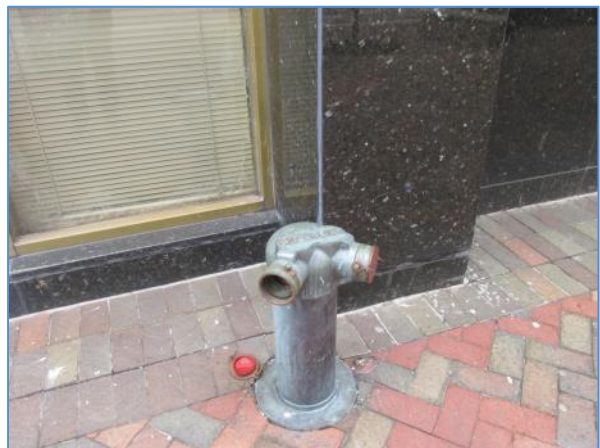
Stand pipe near the pedestrian entrance on the west side of the building
