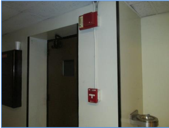
Pull station, strobe and audible alarm in the Lower Lobby
