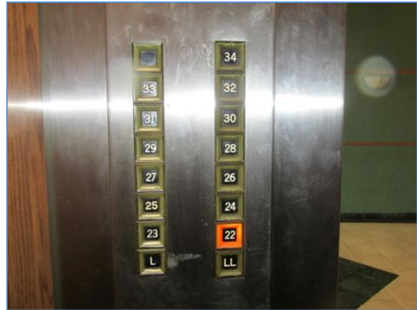
Panel in an elevator serving the upper floors
