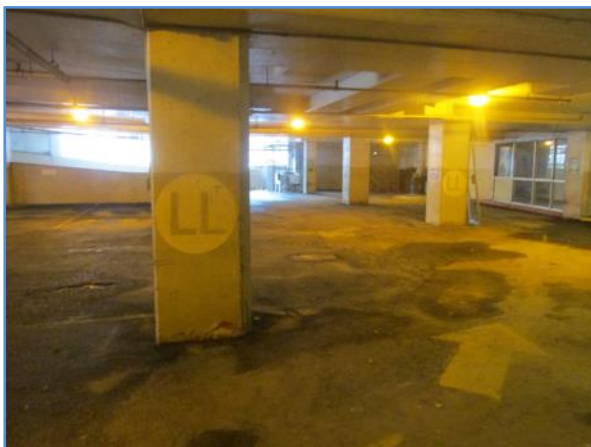
Deteriorated pavement conditions at the lower lobby level of the parking garage
