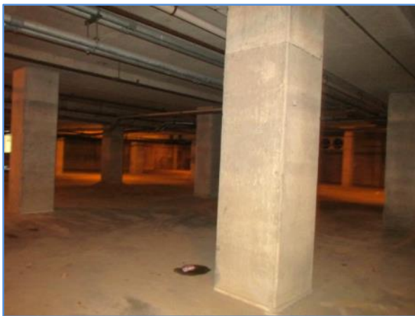
Reinforced concrete columns and floor in the lower level of the parking garage/basement
