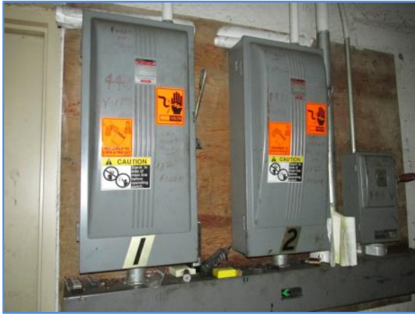
Electrical panels in the elevator equipment room
