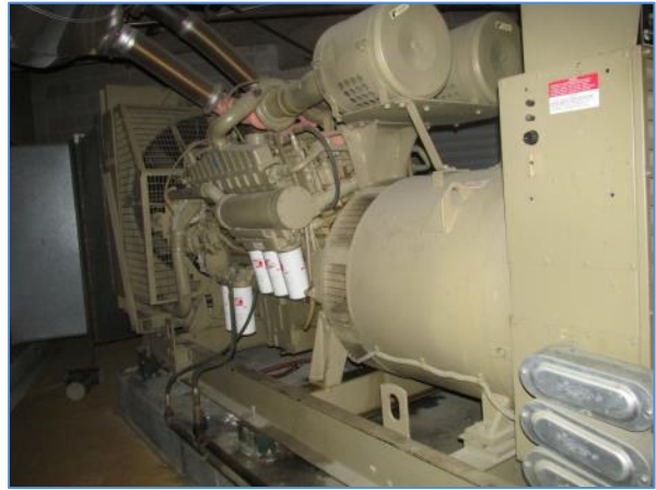
The inactive emergency generator in the basement level of the parking garage
