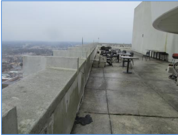
Concrete coping and concrete panels at the outdoor seating area for the rooftop lounge
