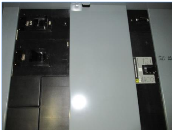
Typical electrical panel in the basement electrical room
