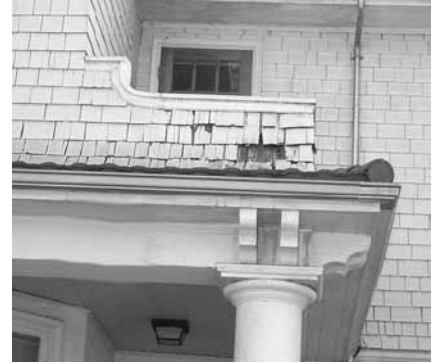
Do not remove damaged materials that can be repaired. In this case, loose shingles may be re-secured while missing ones may be replaced.
