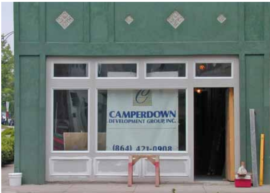
Retain the original shape of the transom when reconstructing a missing one.
