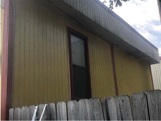
Window to be replaced and awning to be added.
