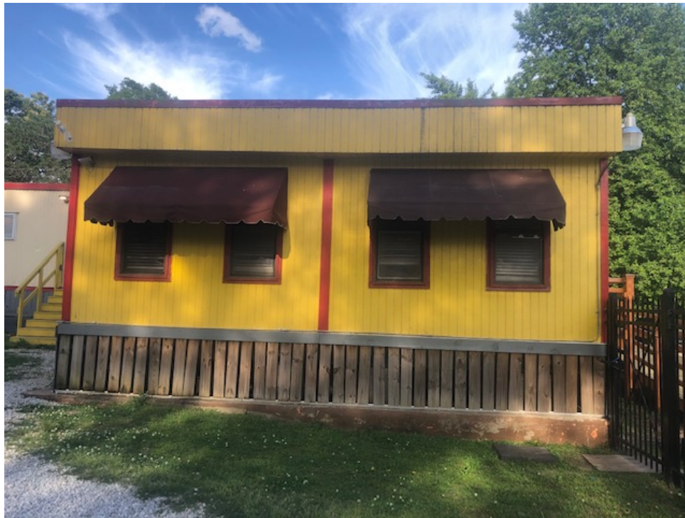
Windows and awnings to be replaced.
