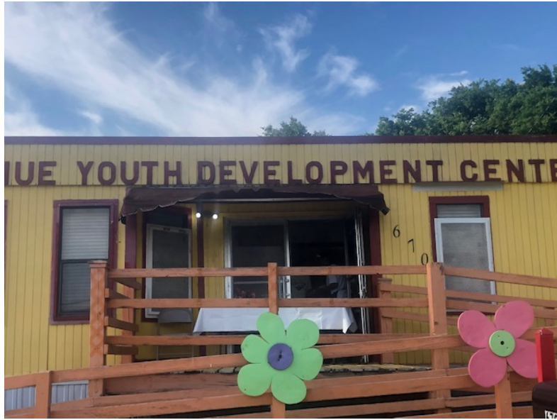
Front door to be replaced and windows. Awning to be replaced.
