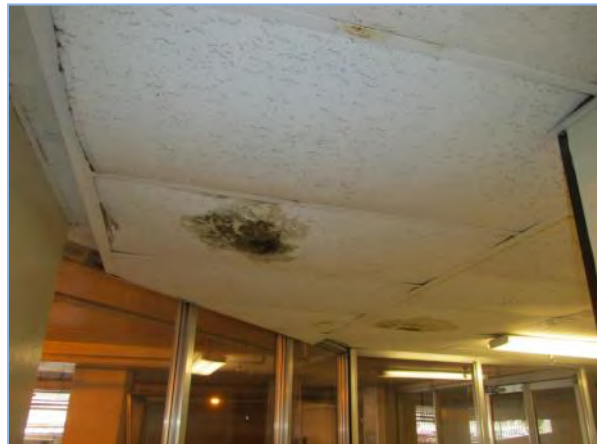
Small area of water damage in the ceiling
