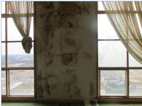
Water damage due to window leaks on an upper floor
