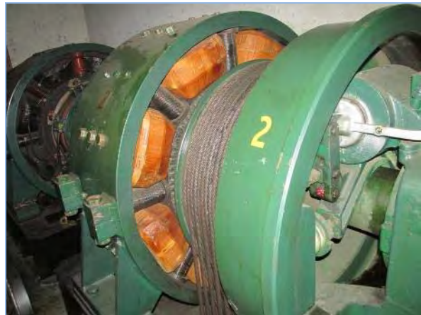
View of elevator equipment in the upper floor mechanical room
