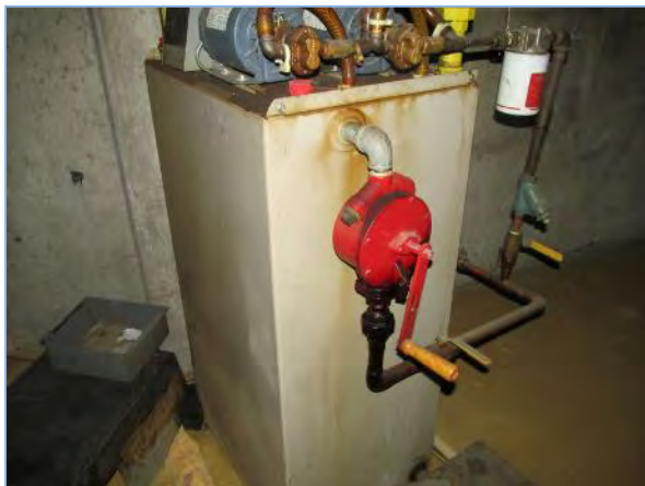
View of the diesel fuel AST (day tank) within the generator room
