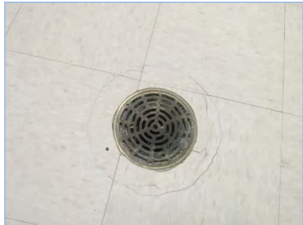
View of a typical onsite floor drain
