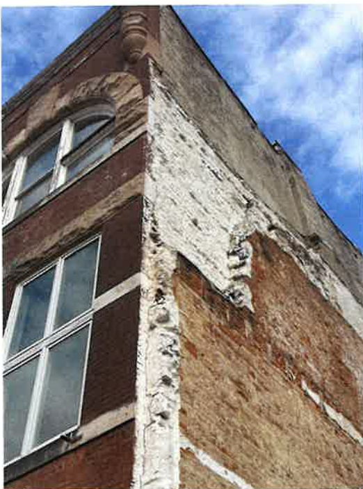
Remnant wall to the south appears to have been partially removed but remains largely intact and exposed to weather.
