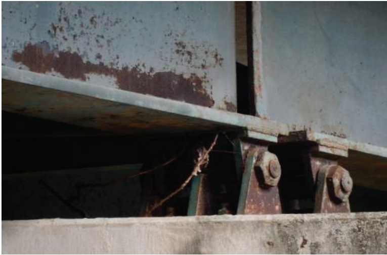
Figure A.08 Steel Paint Deterioration
