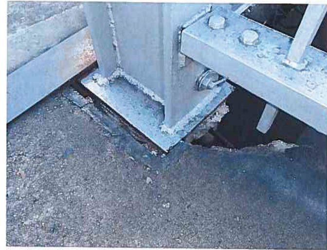
Northwest rail has minor impact damage at northeast end with minor spalling at base of a few rail posts
