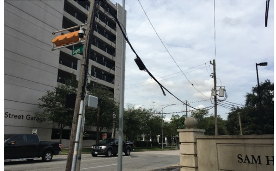
Figure A.01 Overhead Lines at Bagby and Dallas Street
