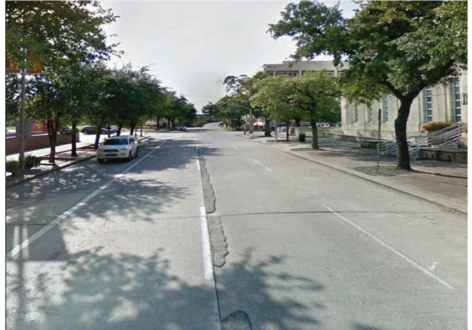
Figure A.02 Concrete Panels Settlement along McKinney Street east of Bagby Street
