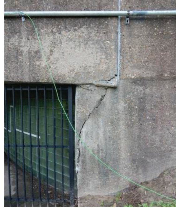
Figure A.17 Moderate Cracking in Retaining Wall
