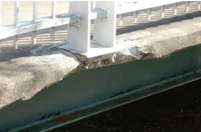
Figure A.09 Concrete Spall at Rail Post on West Sidewalk
