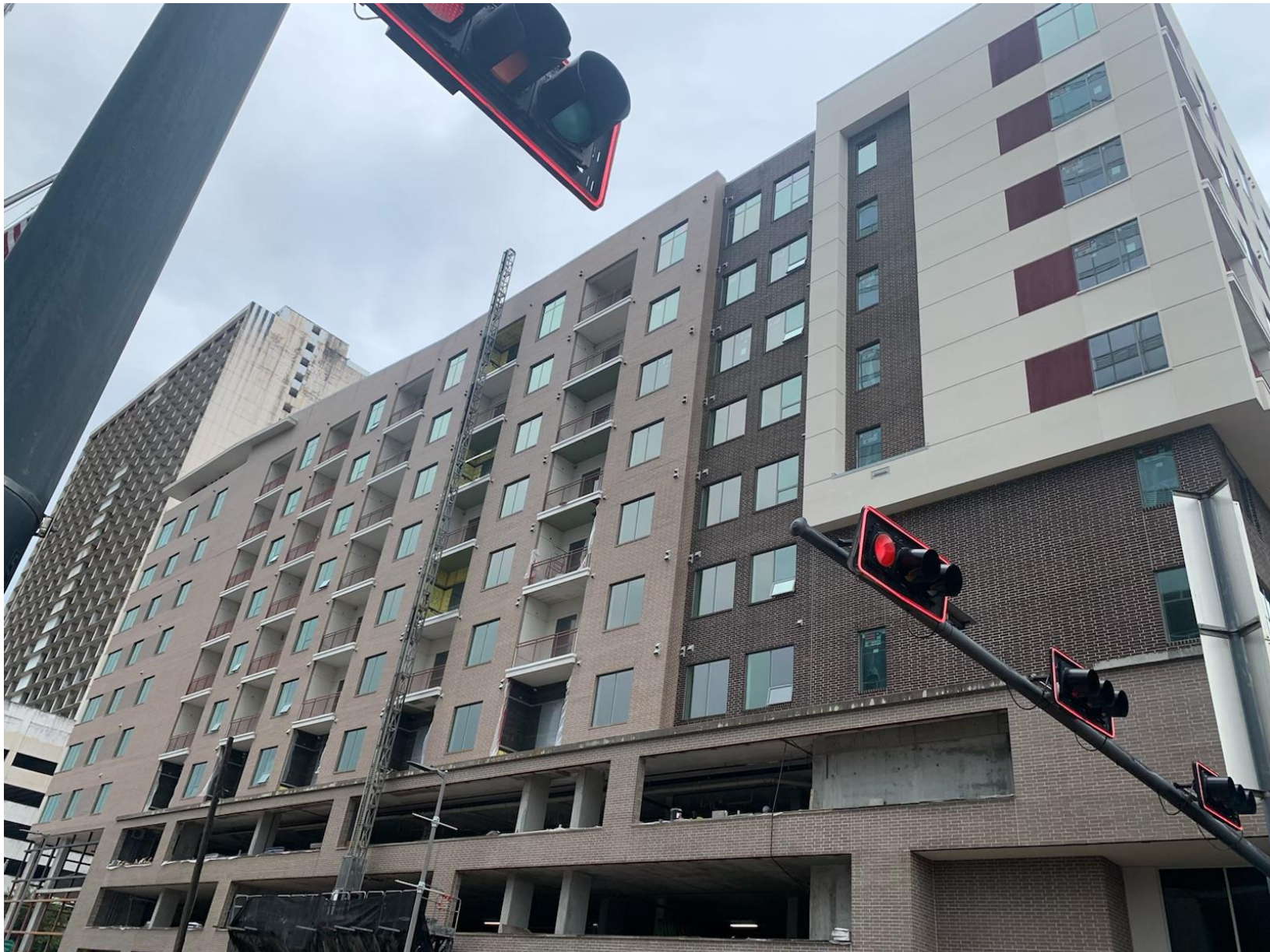
1810 MAIN STREET FAIRFIELD RESIDENTIAL PROGRESS PHOTO VIEW FROM CORNER OF MAIN STREET AND ST JOSEPH PARKWAY (AUG. 5, 2022)
